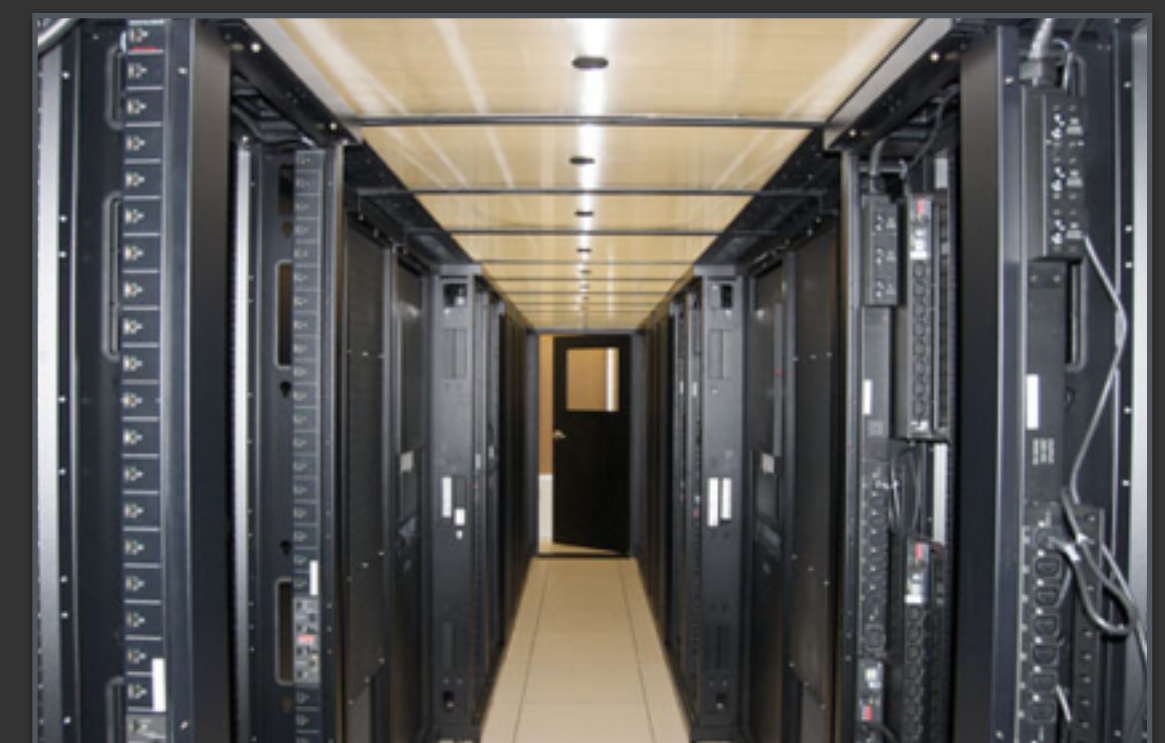
On-campus Parallel Data Lab Datacenter
