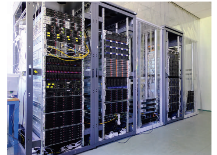
>> Fig. 2: Computational clusters in the server room at Warsaw.
