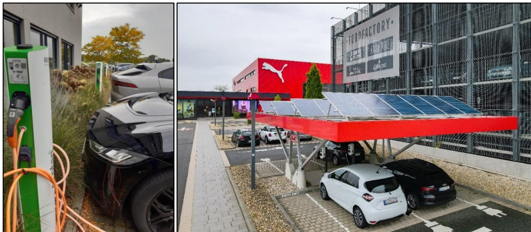
Charging station for electric cars at Stichd headquarters and at the PUMA headquarters in Herzogenaurach.
