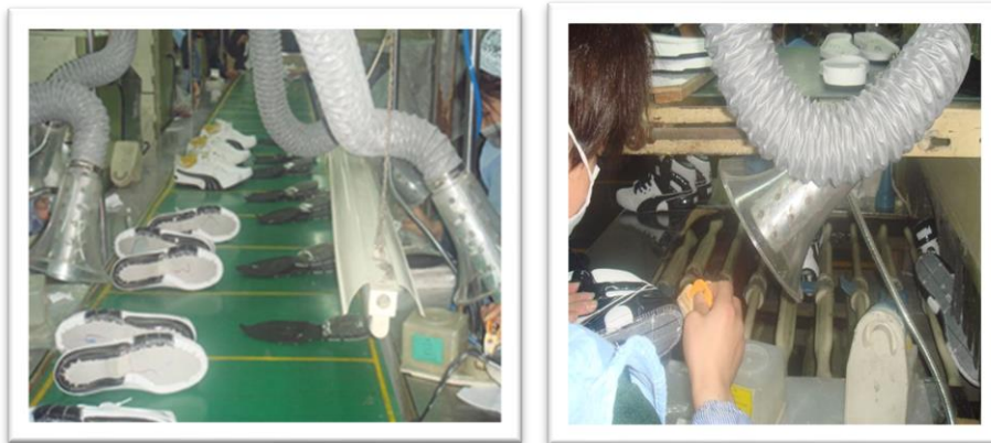
Figure 13: example of Local Exhaust Ventilation system
