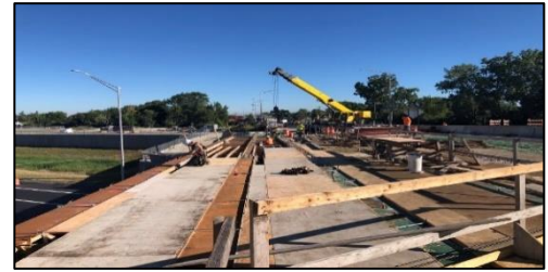
Construction of the 88th/Cork Avenue Bridge over the Central Tri-State Tollway (I-294) near Justice
