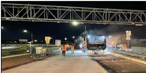
Ramp pavement repairs at the Reagan Memorial Tollway (I-88)/Illinois Route 31 interchange near North Aurora
