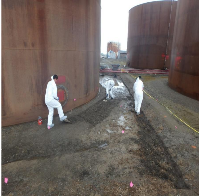
At the Eskimo's Inc. facility in Barrow, Alaska a pressure relief valve failed releasing an estimated 9,000 gallons of unleaded gasoline into the tank farm's secondary containment. Responders use non-sparking tools to remove contaminated gravel from the secondary containment area, July 19, 2017 (Photo/ ADEC)
