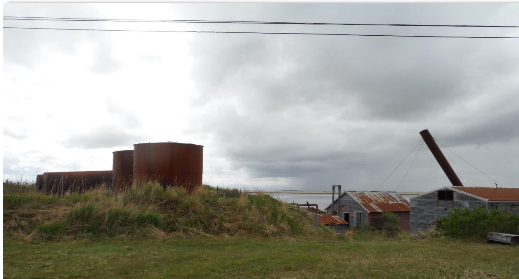
Alaska Packers Association cannery in Ugashik, Bristol Bay Alaska - View of four above ground storage tanks and former power house building at the Ugashik cannery. View of four above ground storage tanks and former power house building at the Ugashik cannery (Photo Erin Gleason/ADEC)
