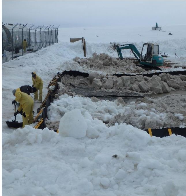
At the Savoonga Native Store Tank Farm an estimated 22,000-gallon release of diesel fuel was released to the Savoonga tank farm secondary containment area and surrounding environment. Responders move contaminated snow and ice to the temporary containment area, April 23, 2018 (Photo/ ADEC)
