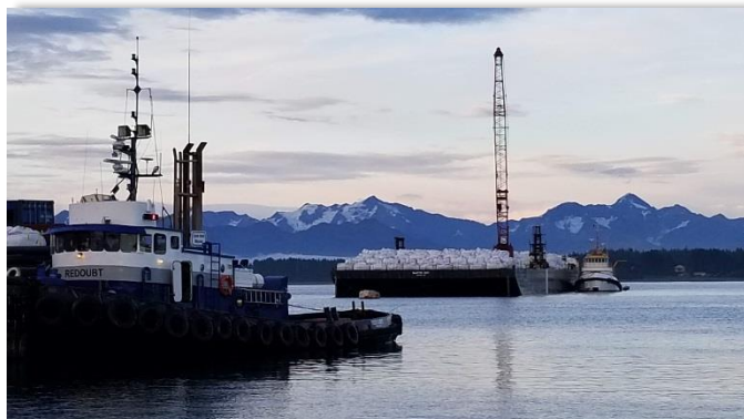
Former Point Carrew Garrison Yakutat, Alaska FUDS Contaminated Soil Loaded on Barges for Disposal (Photo/USACE)
