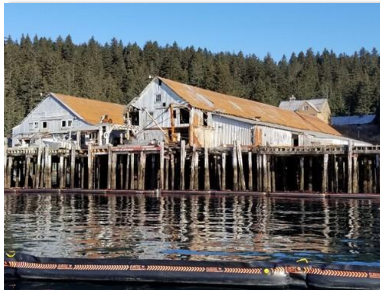
Port Williams Cannery on the south side of Shuyak Island, Alaska, March 29, 2018. The collapse of a fuel bladder with up to 3,000 gallons of mixed fuels released products into the Bay and along the adjacent shoreline. Response Contractor Alaska Chadux deployed 3,340 feet of boom and absorbents in the Bay (Photo/Jade Gamble, ADEC Responder)
