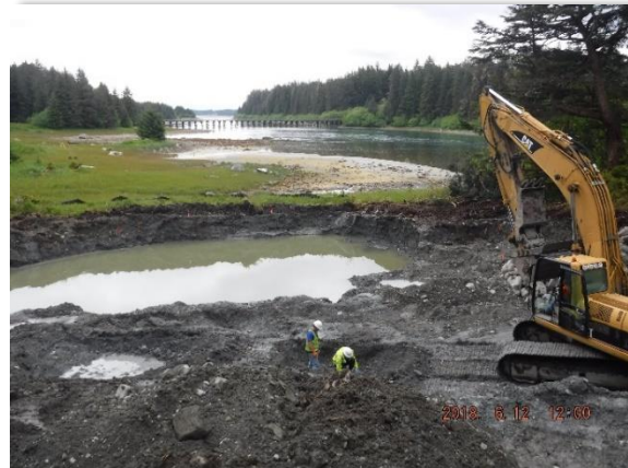
Former Point Carrew Garrison Yakutat, Alaska FUDS 50,000-gallon Aboveground Storage Tank excavation, 2018(Photo/ USACE)
