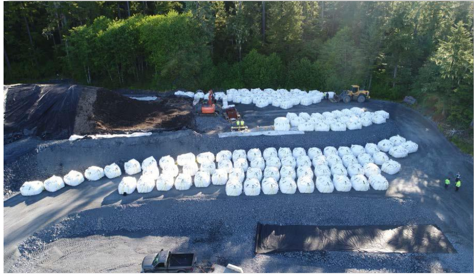
A former salvage yard in Wrangell Alaska, June 2018 showing treated lead contaminated soil being loaded into 8-cubic yard flexible intermodal bulk containers for transport and disposal out of state. (Photo/NRC)
