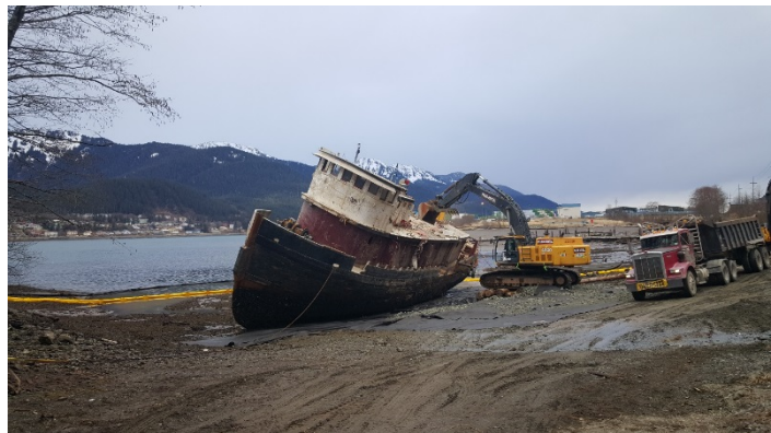
Deconstruction of the Tug Challenger after sinking and subsequent raising, February 2016 (Photo/DEC)
