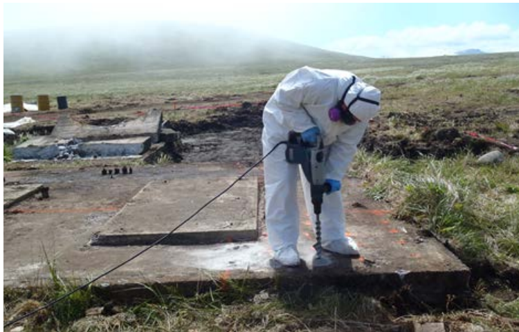
Generator building concrete pad sampling and demolition at Cape Kadugnak FUDS (Photo/Bethel Services, Inc. – TLI Solutions, Inc. Joint Venture)
