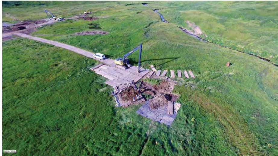
Armored long-reach excavators performing mass excavation of MEC disposal area. UXO technicians are visible in the foreground sorting excavation spoils (Photo/CB&I Federal Services)
