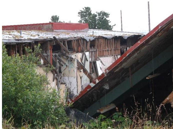
Collapsed former Kake elementary school. (Photo/DEC- Danielle Duncan)
