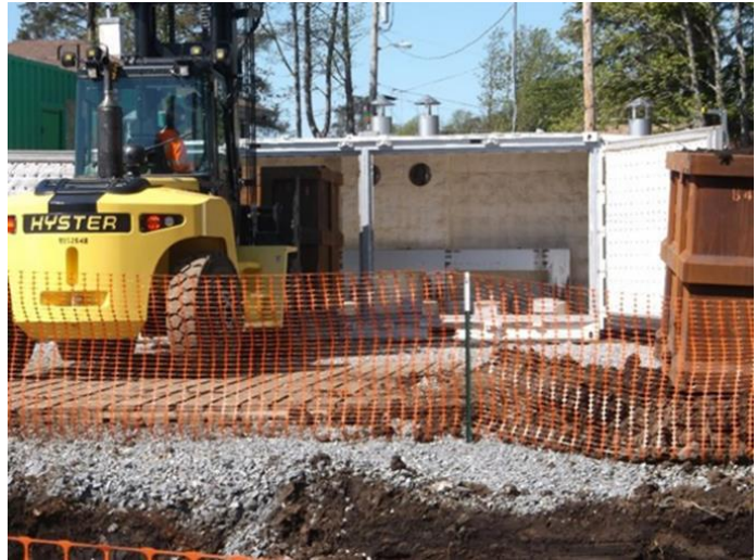
Excavation and high temperature (Reterro) treatment of petroleum contaminated soils. (Photo/DEC- Danielle Duncan)
