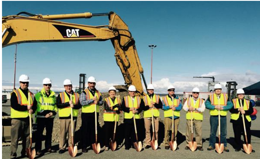
Delta Western and Port Officials break ground for the new methanol terminal (Photo/DEC)
