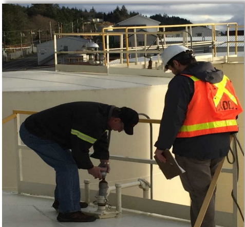
Cronley Fuels LLC, Ketchikan terminal tank farm overflow prevention testing November 29, 2018 (Photo/DEC)
