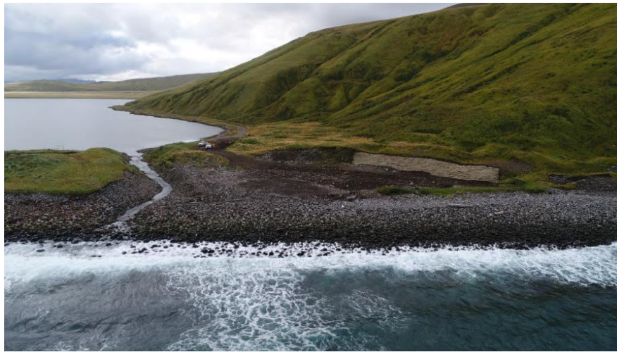
Andrew Lake Spillway (landfill that contained munitions) removal area end of 2017 field season. Metal waste shipped to Washington for recycling. Munitions destroyed on site by detonation (Photo/CB&I Federal Services)
