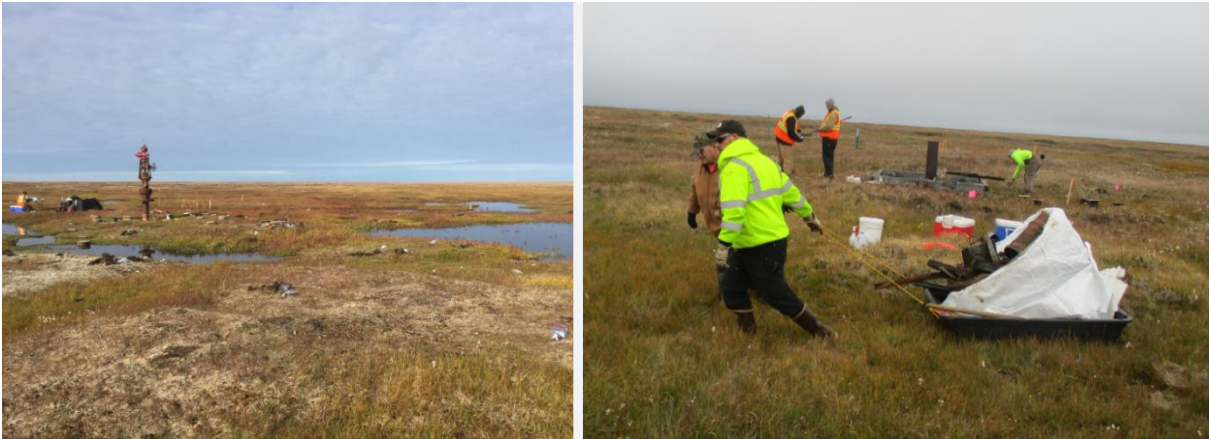
LEFT - Field screening of bagged samples at Iko Bay #1 following sampling during fall 2016 field season work. RIGHT - Removal of surface debris from Avak #1 to nearby road for disposal (Photos/Marsh Creek LLC)
