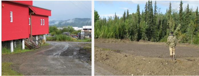
LEFT - Section of the road by Kaltag School that was excavated and backfilled. RIGHT - Plot of contaminated soils from the Kaltag School being treated by phytoremediation, 2015 (Photo/DEC)
