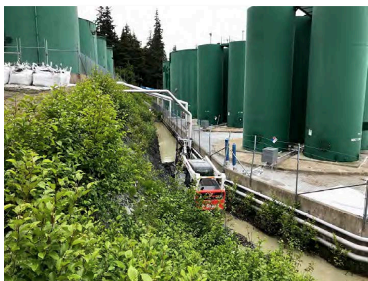
A cleanup crew removes petroleum-impacted soil from the drainage swale in June 2020 after the Delta Western Haines Facility Tank 1 Release. Supersacks with impacted soil can be seen in the upper left. (Photo/DEC)
