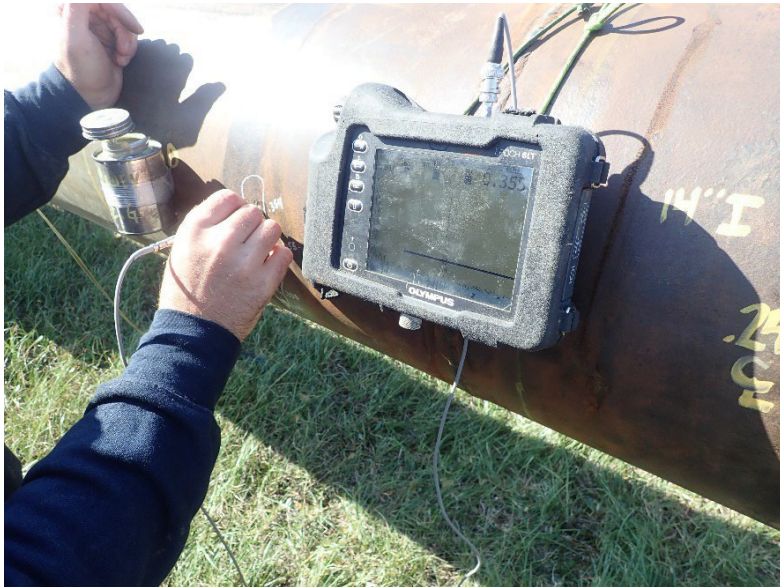
Photo: Pipeline inspection crews performing external corrosion inspections using an ultrasonic pencil probe on 3-phase flowline 02E between DS-2 and Flow Station 1.
