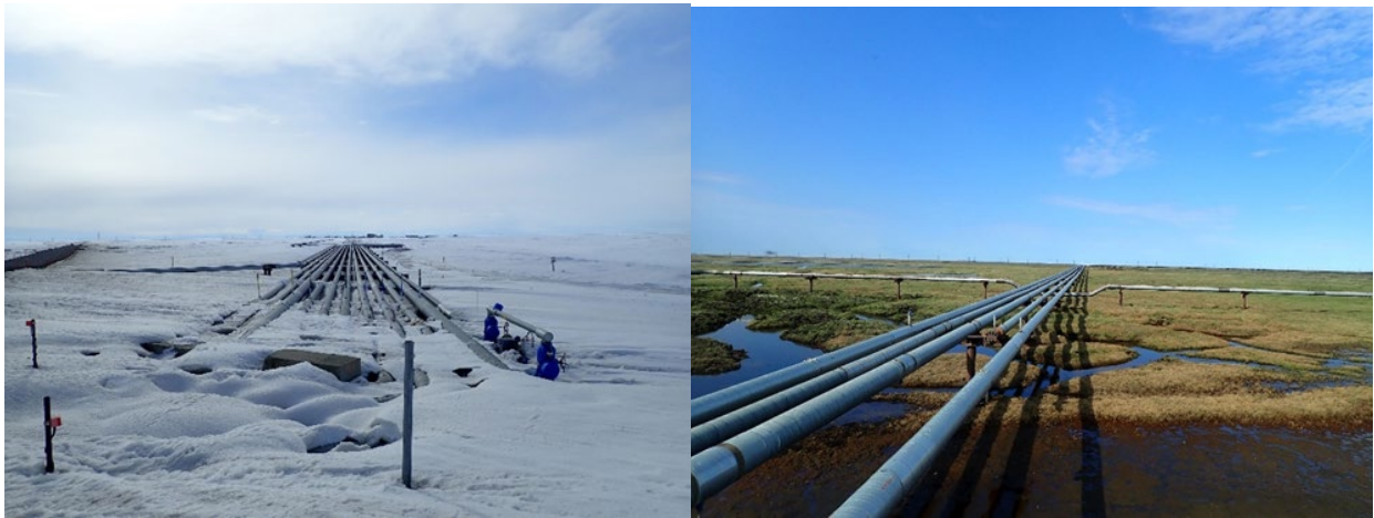
Pipelines in the Prudhoe Bay field, crossing the Sagavanirktok River (left) and in the Kuparuk River field, crossing the tundra in the vicinity of CPF-3 (right)
