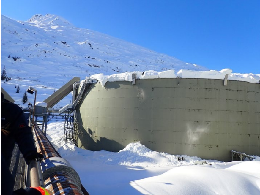
A tank at the Valdez Marine Terminal with damaged vents and accumulated snow on the roof
