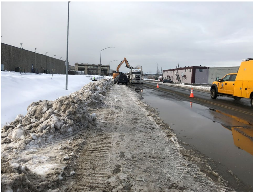
Clean up work on the Alaska Airlines Facility Maintenance AFFF release along the road way
