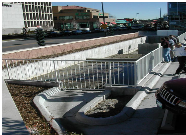
EXHIBIT 6.80 DIFFICULT BMP MAINTENANCE ACCESS
