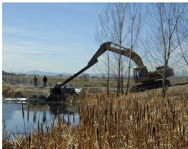
EXHIBIT 6.79 SEDIMENT REMOVAL FROM A FOREBAY AT THE REGIONAL SHOP CREEK BMP SYSTEM
