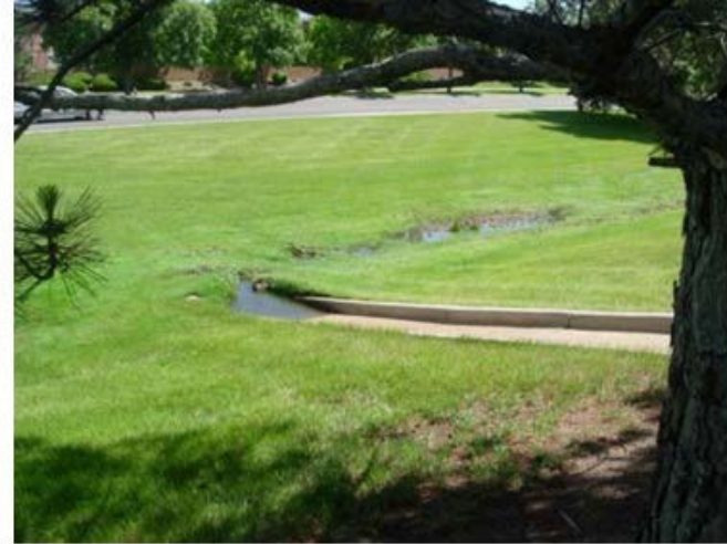
Inflow Point has erosion and sediment build-up Maintenance required
