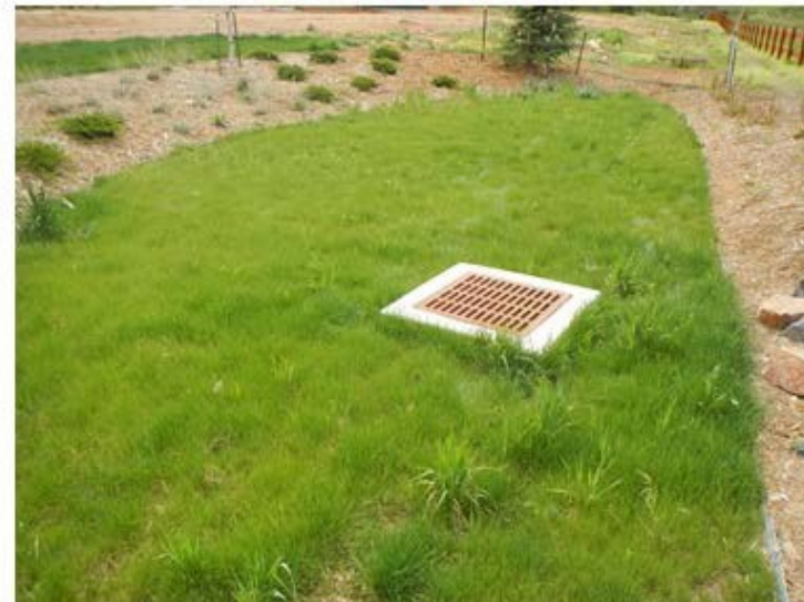
Rain Garden with healthy vegetation and no sediment No immediate maintenance required
