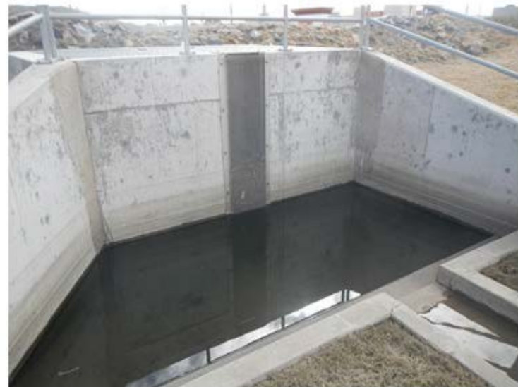
Micropool is clean – no debris, vegetation, excess sediment No immediate maintenance required
