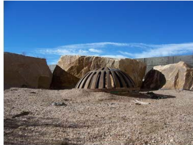
Outlet Structure installed too low (cross-check with design) Maintenance required
