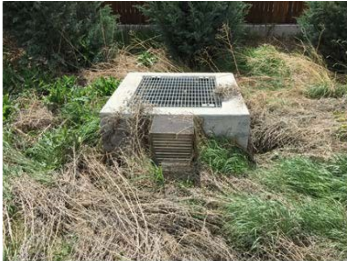
Outlet Structure with excess vegetation growth Maintenance required
