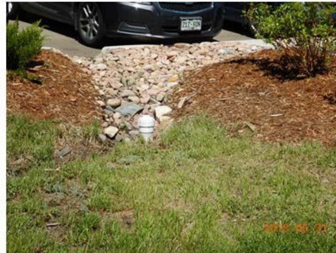
Inflow Point operating correctly No immediate maintenance required
