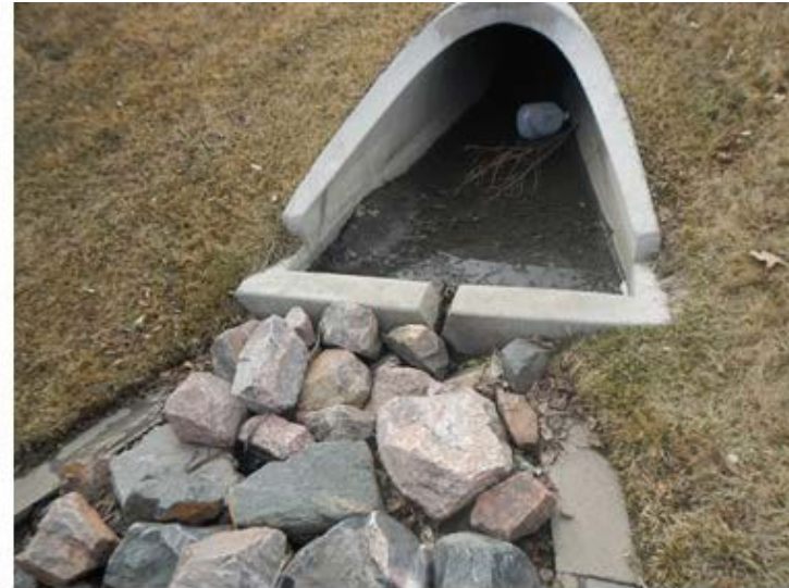
Sediment build-up and forebay outlet is clogged Maintenance required
