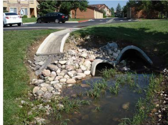
Erosion is present and rip-rap displacement has occurred Maintenance required
