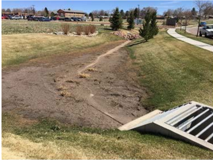
Excess sediment accumulation in basin area Maintenance required
