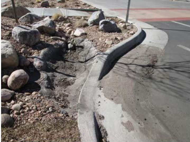
Outlet of forebay is clogged/blocked causing runoff bypass Maintenance required
