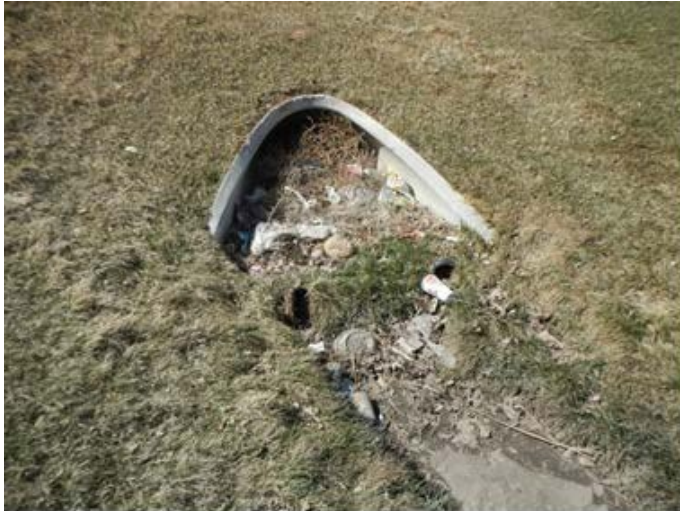
Inlet is clogged with trash and debris Maintenance required
