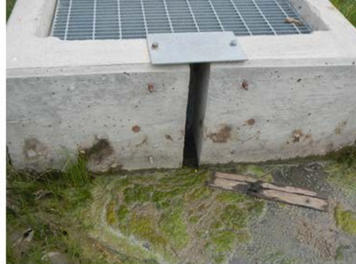
Well screen is missing from outlet structure Maintenance required
