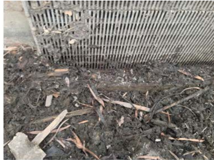
Outlet screen is clogged due to debris in micropool Maintenance required
