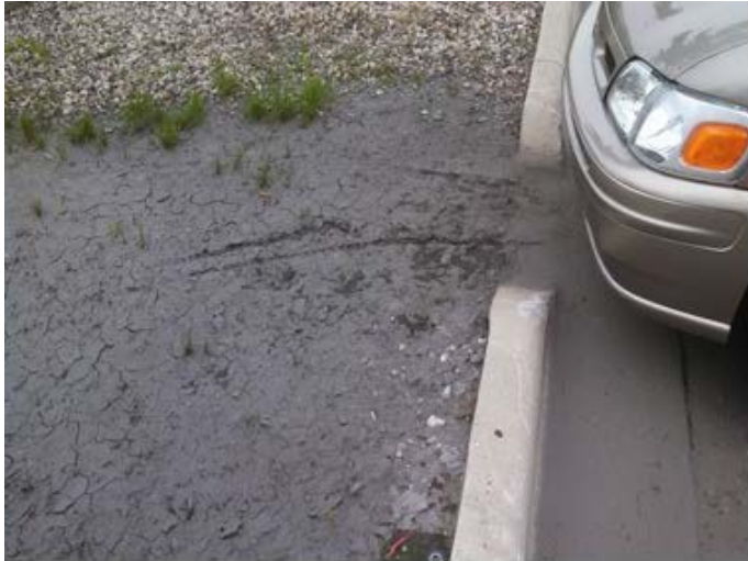
Curb-cut inlet with excessive sediment build-up Maintenance required
