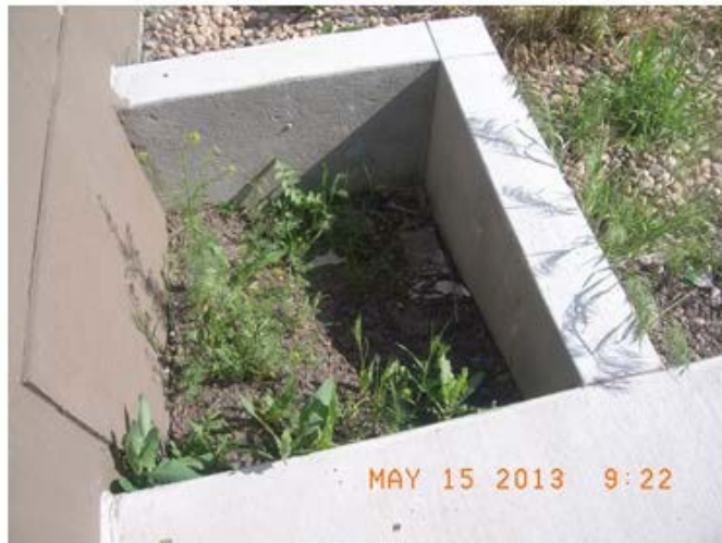
Outlet Structure clogged with sediment Maintenance required
