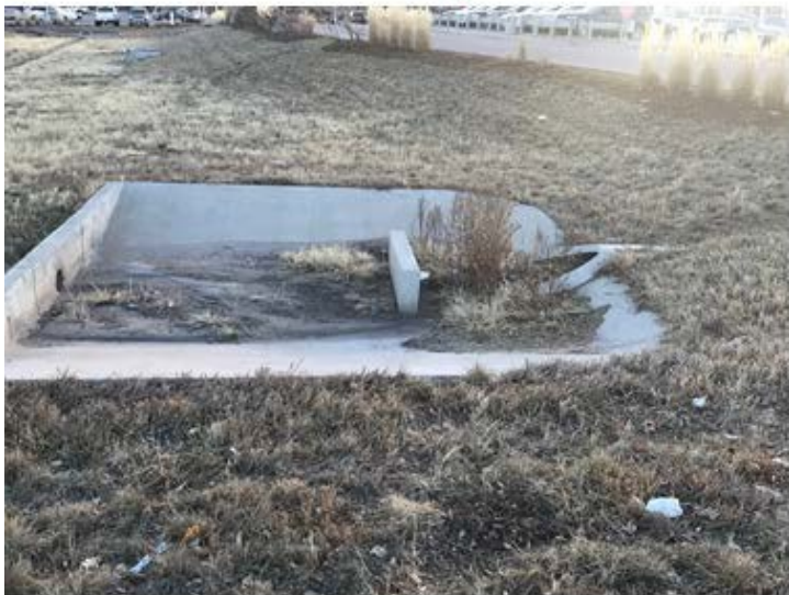
Sediment accumulation and vegetation growth Maintenance required
