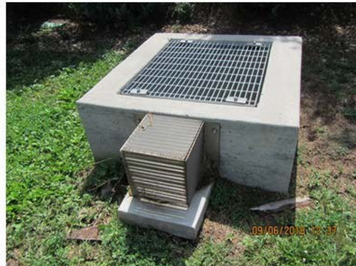
Outlet works clear of debris and properly installed No immediate maintenance required
