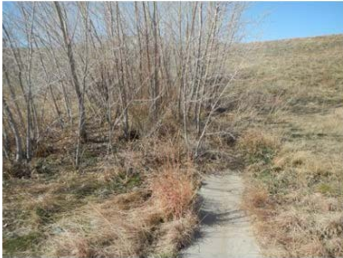
Woody debris buildup in basin area Maintenance required
