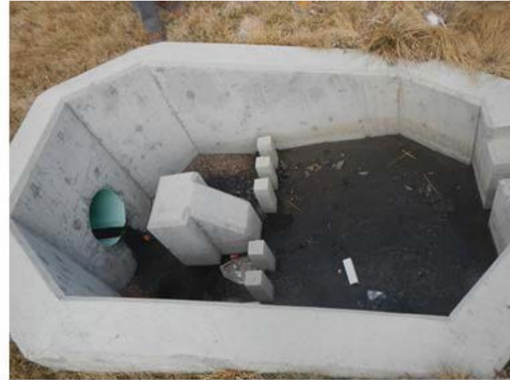
Trash and sediment accumulation in forebay Maintenance required
