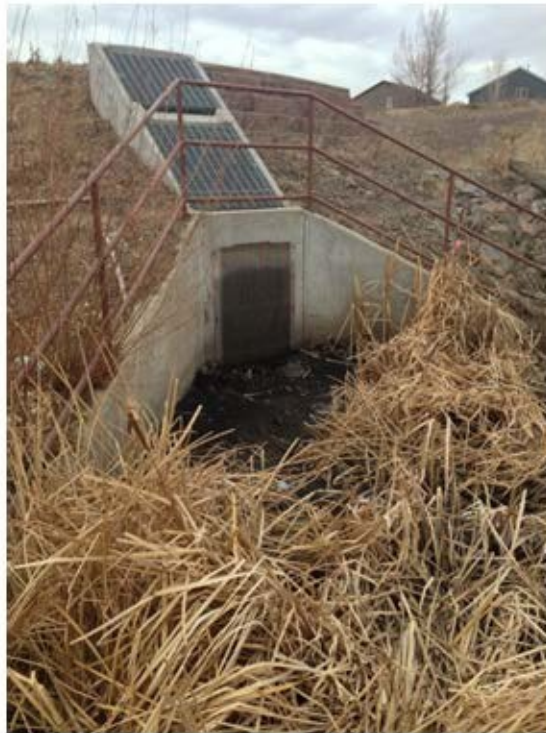
Micropool with excess sediment buildup and vegetation growth Maintenance required
