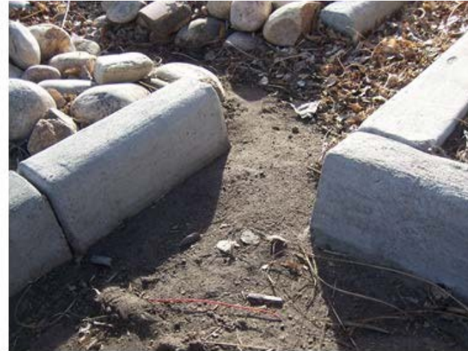
Inflow Point with sediment and debris accumulation Maintenance required
