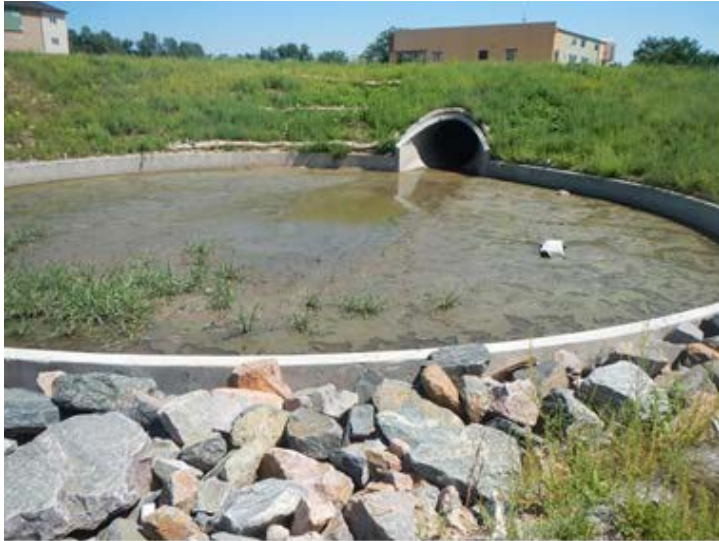
Forebay is full of sediment, standing water and vegetation Maintenance required
