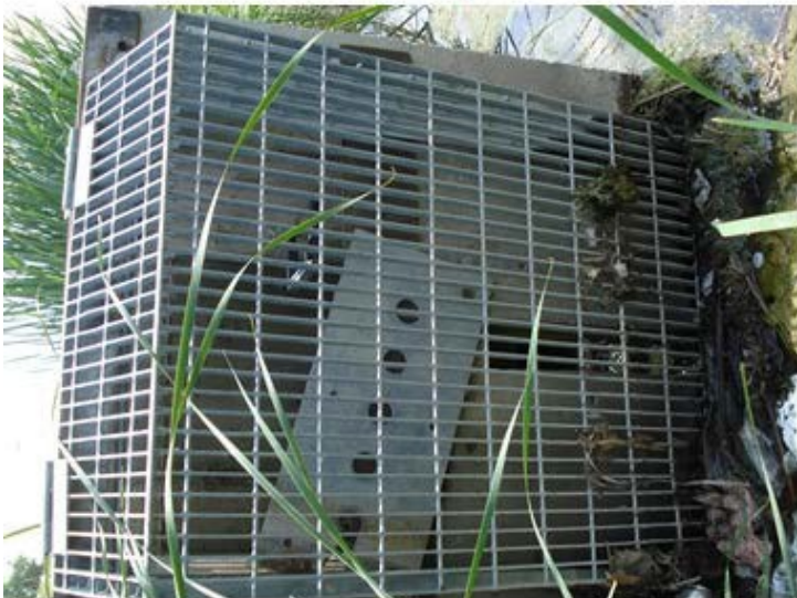
Orifice plate is not secure/dislodged Maintenance required
