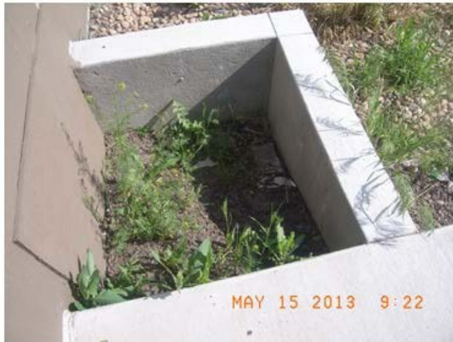
Outlet Structure clogged with sediment Maintenance required
