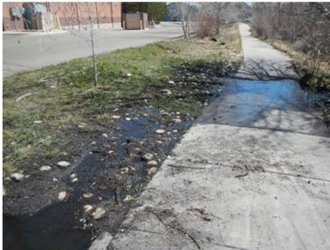
Inflow Point with erosion and sediment build-up Maintenance required
