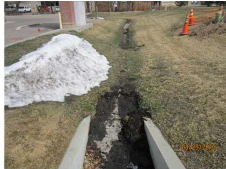
Sediment build-up in trickle channel due to snow storage Maintenance required
