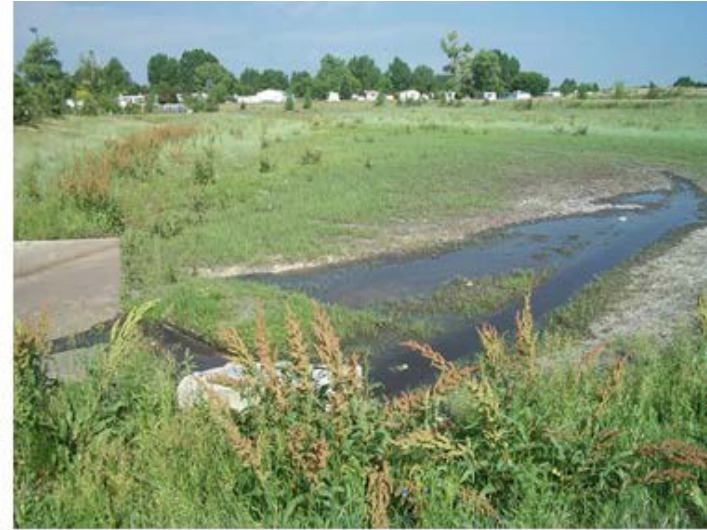
Standing water issues in basin area Maintenance required
