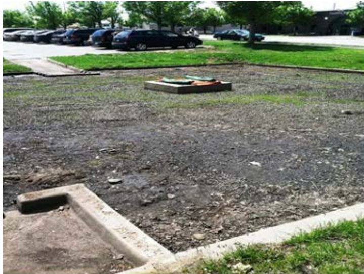
Sand Filter media with excessive sediment build-up Maintenance required
