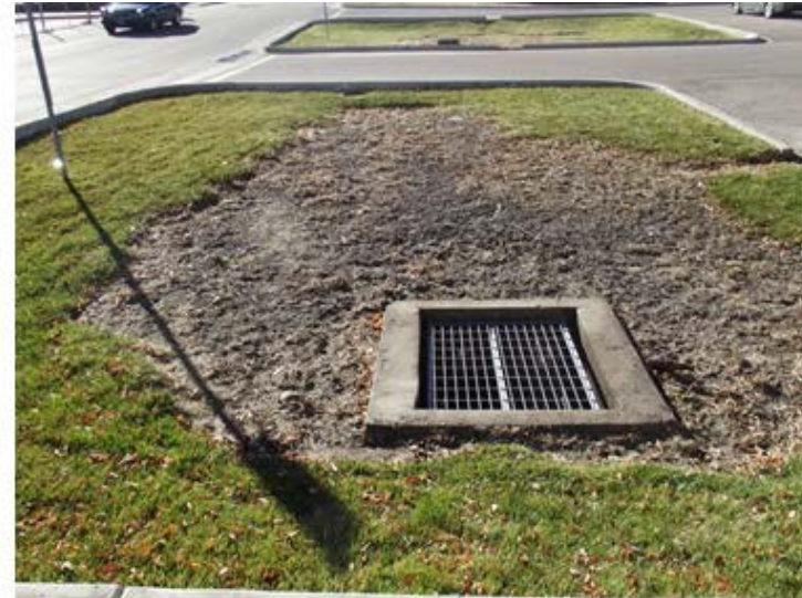
Rain Garden with dead vegetation on filter media surface Maintenance required
