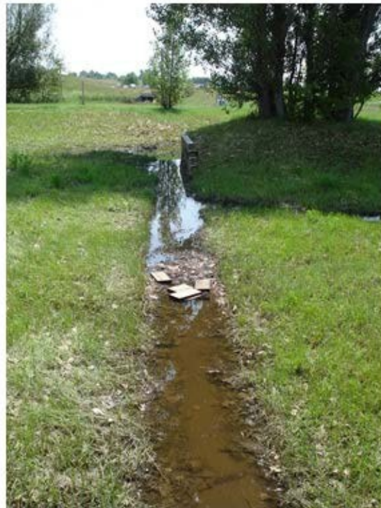
Trickle channel clogged with debris and sediment accumulation Maintenance required
