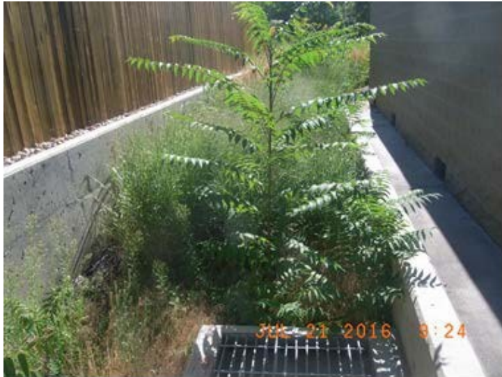
Woody/overgrown vegetation in rain garden Maintenance required
