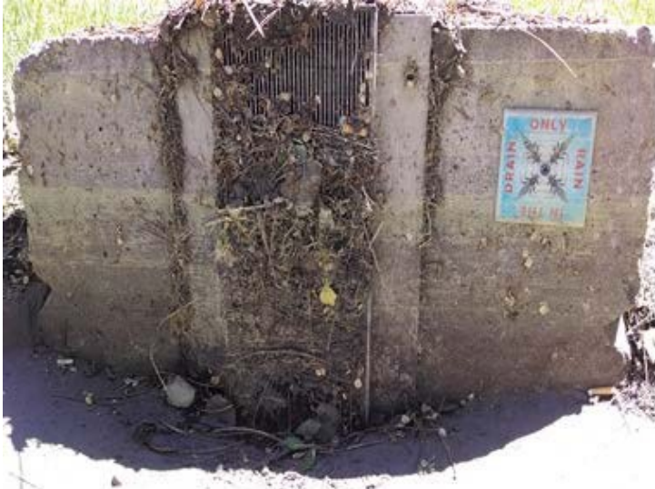
Trash rack and well screen are clogged with debris Maintenance required
