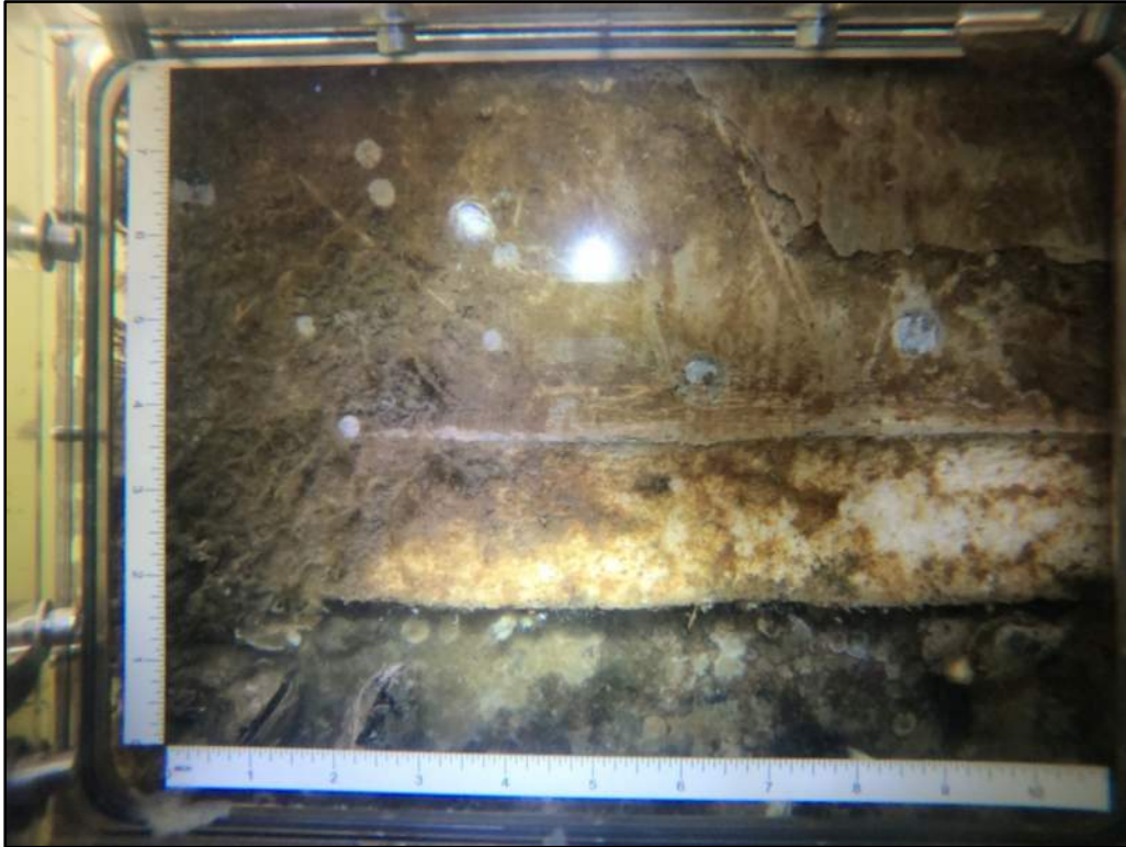
Photo 23: Typical Condition of Square Epoxy Jacket Underwater (Bent 130, Pile 4 Shown).
