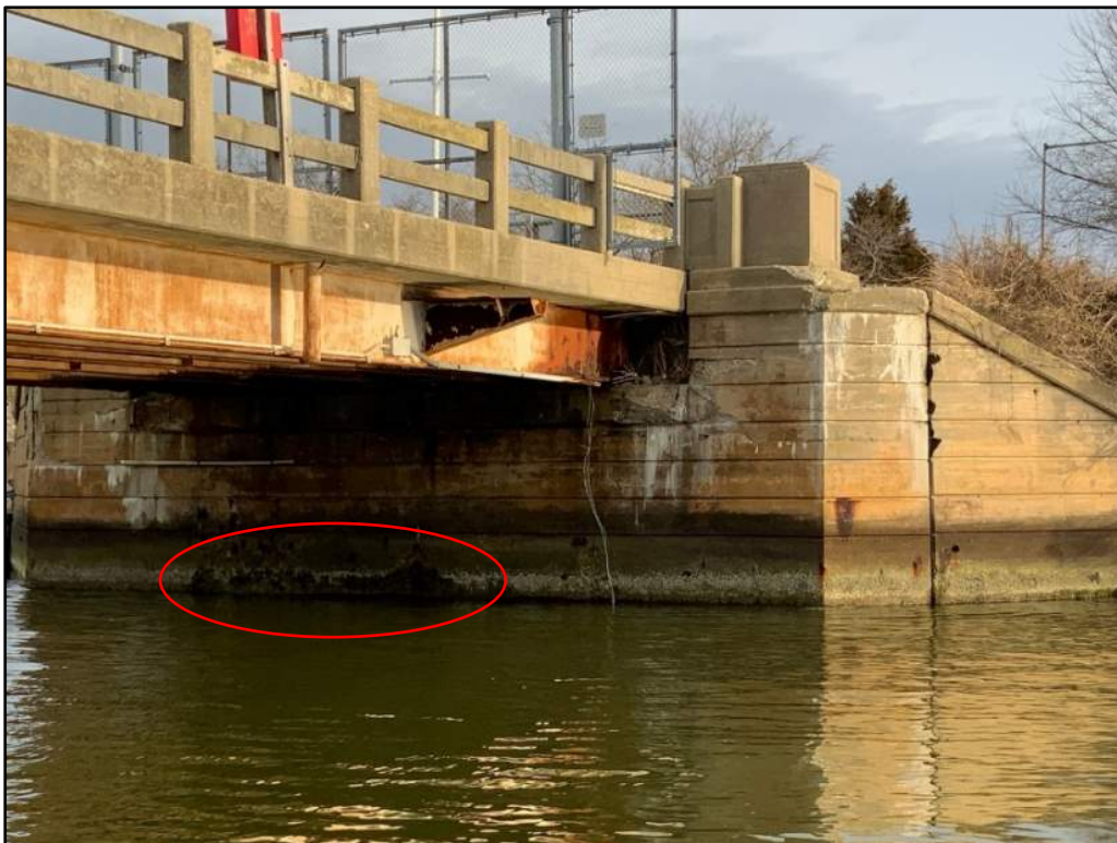
Photo 34: North Abutment (Bent 151), Spalling at the Waterline.
