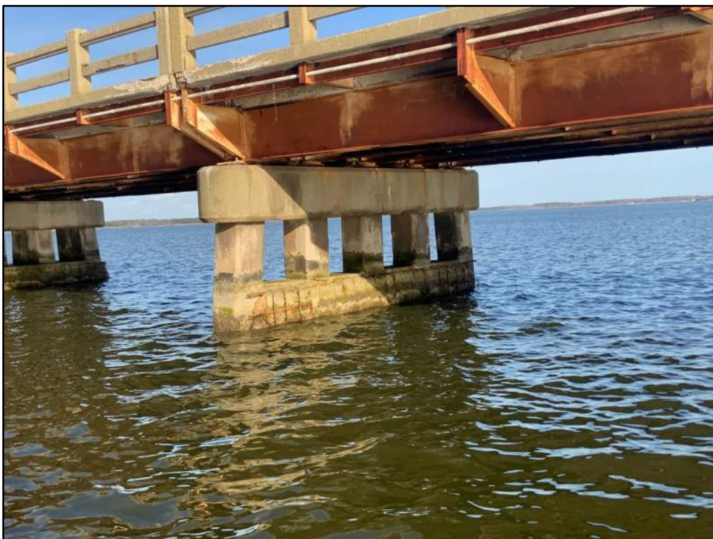
Photo 14: Typical Missing Strut on East and West Faces (Bent 39 Shown).
