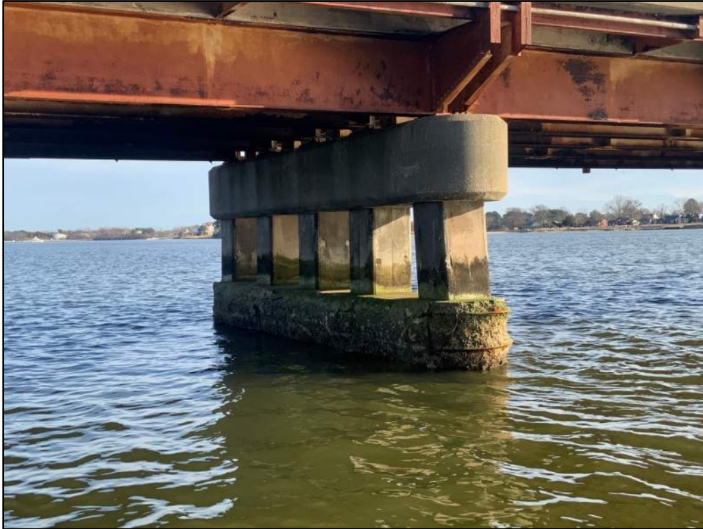
Photo 15: Typical Spalling and Exposed Reinforcement on West and East Ends of the Strut (Bent 30 Shown).
