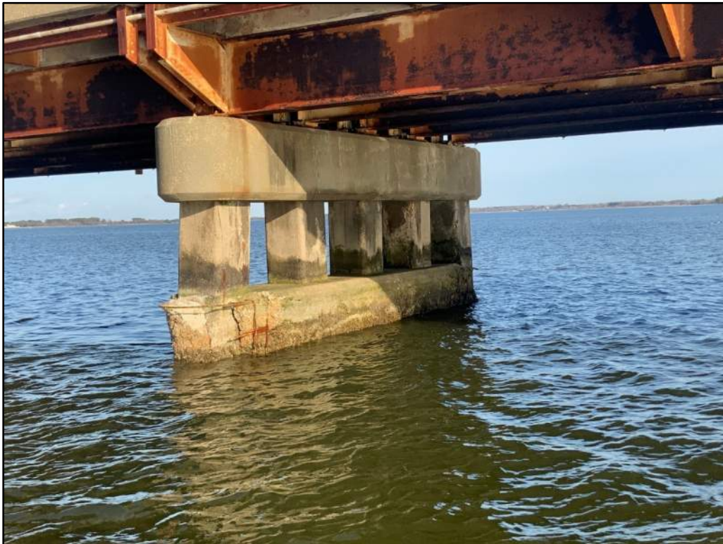
Photo 13: Typical Spalling and Exposed Reinforcement on Strut (Bent 28 Shown).
