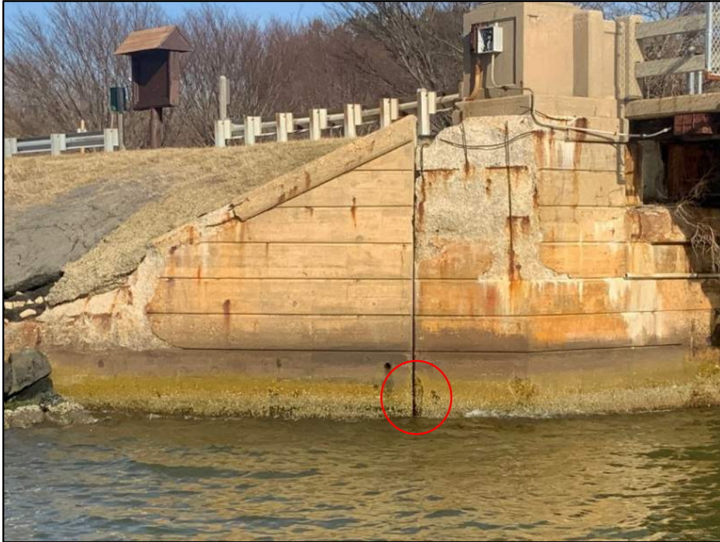
Photo 33: North Abutment (Bent 151), Spalling at the Waterline.
