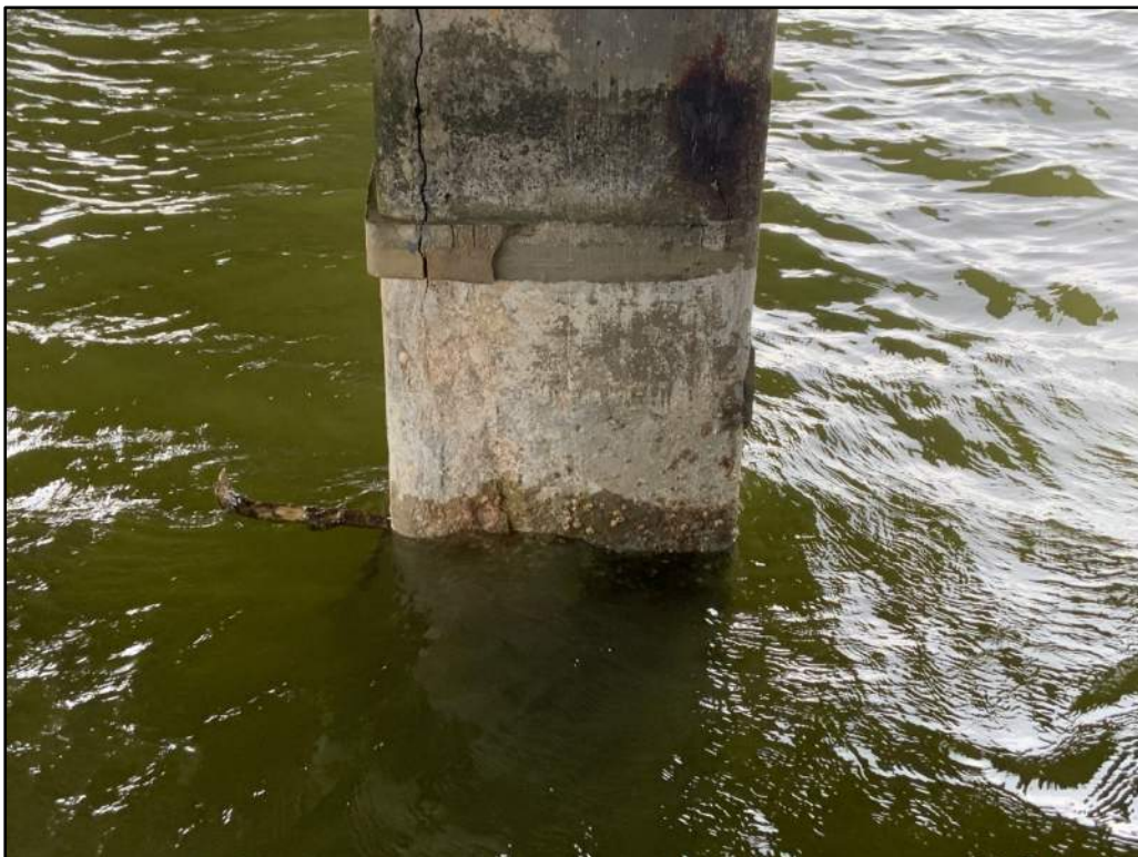
Photo 24: Bent 130, Pile 2, Missing Jacket and Abrasion in the Tidal Zone.
