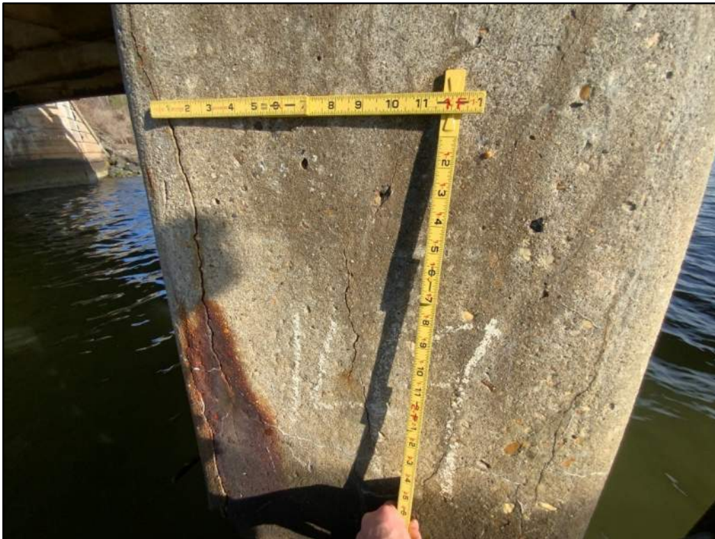
Photo 18: Typical Vertical Cracking at the Top of Pile (Bent 150, Pile 5 Shown).
