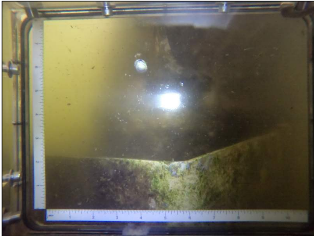
Photo 25: Bent 130, Pile 2, Failed Square Epoxy Jacket (Underwater).
