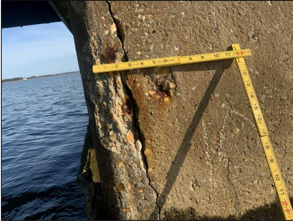
Photo 19: Bent 109, Pile 5, Area of Spalling and Delamination at the Top of Pile.
