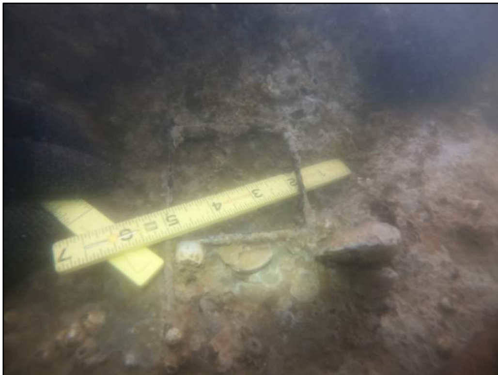
Photo 26: Bent 40, Pile 1, Void at the Top of the Grout Filled Fabric Bag Repair (Underwater).
