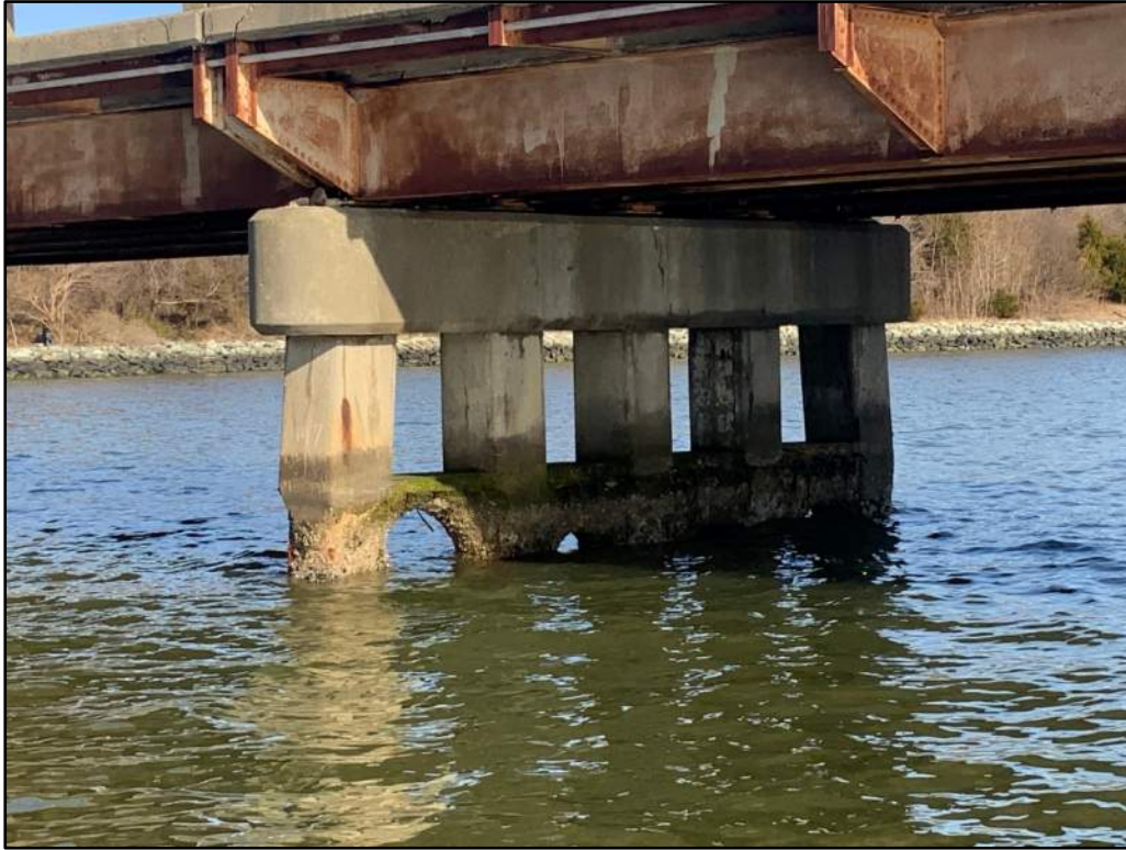
Photo 11: Typical Spalling and Exposed Reinforcement on Strut (Bent 147 Shown).
