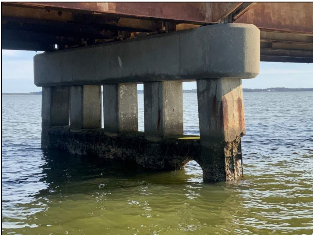
Photo 10: Typical Spalling and Exposed Reinforcement on Strut (Bent 149 Shown).
