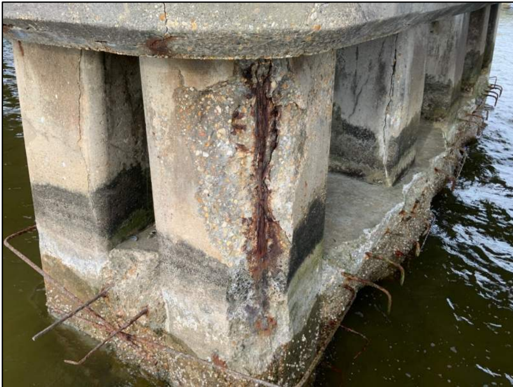
Photo 21: Bent 8, Pile 5, Corner Spall with Exposed and Corroded Reinforcement.
