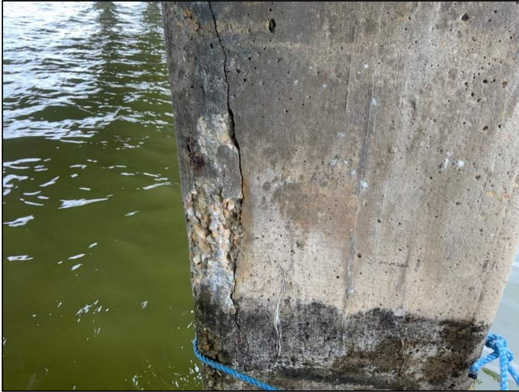
Photo 17: Bent 130, Pile 1, Corner Spall and Delamination.
