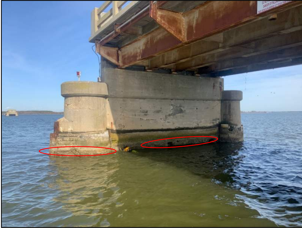
Photo 27: Pier Wall 1 (Bent 56), Scaling and Voids at the Waterline.
