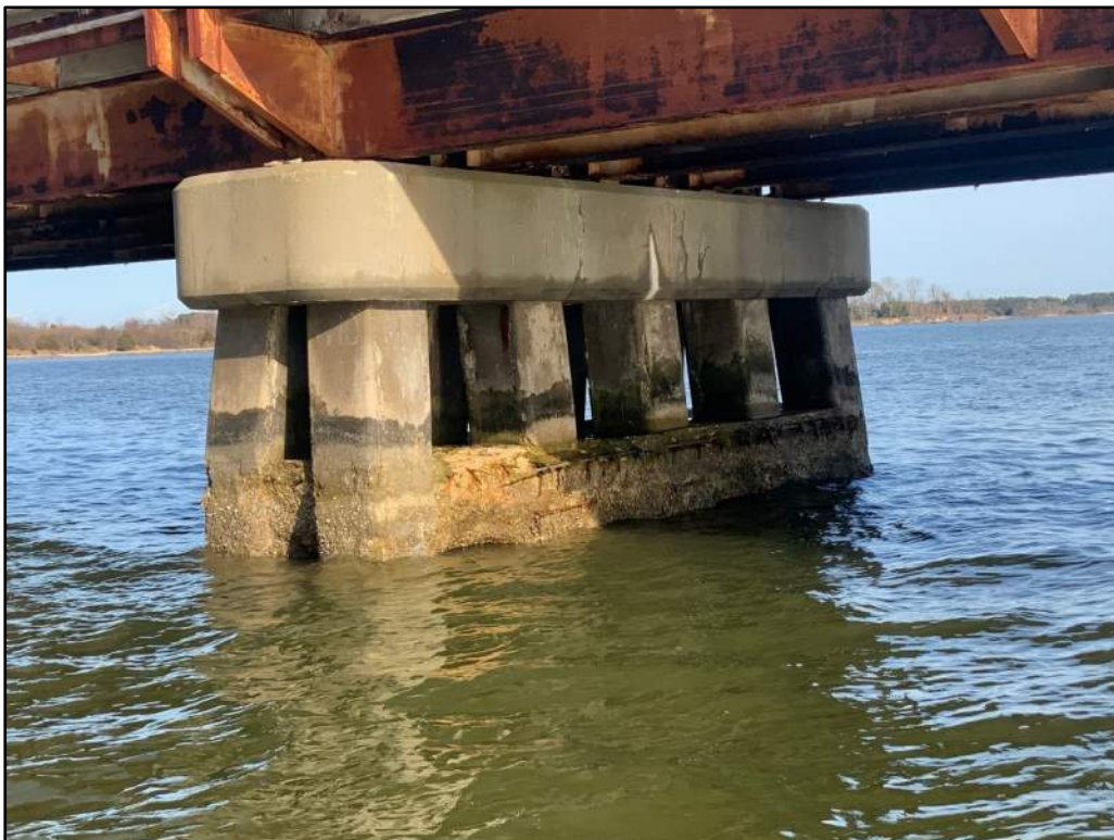
Photo 12: Typical Spalling, Exposed Reinforcement, and Missing West and East Ends on Strut (Bent 111 Shown).
