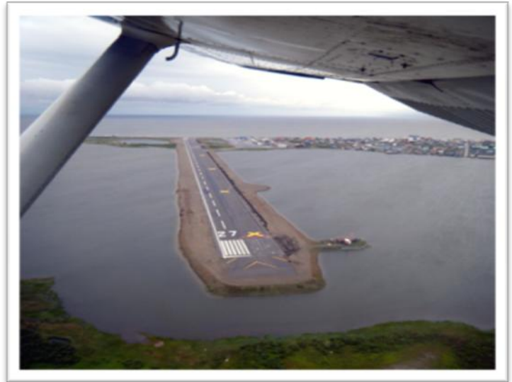
The Kotzebue Airport was able to maintain operations this year even through runway improvements. The airport closed half of the runway during construction.
