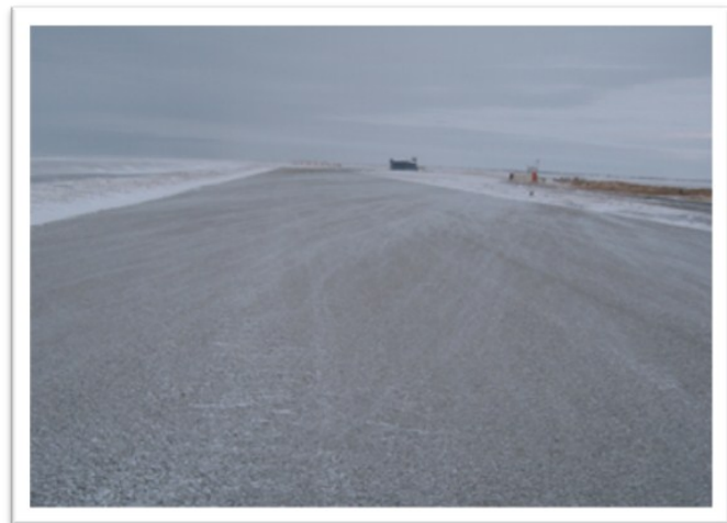
Platinum Runway Extension Project. Engineering work has begun, and the project will be bid this spring with construction set for summer 2013.
