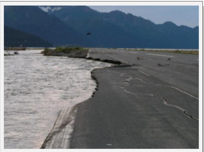
Erosion and overflow from the flooding Resurrection River damaged and temporarily closed the Seward Airport in 2013. (ADOT&PF photo)
