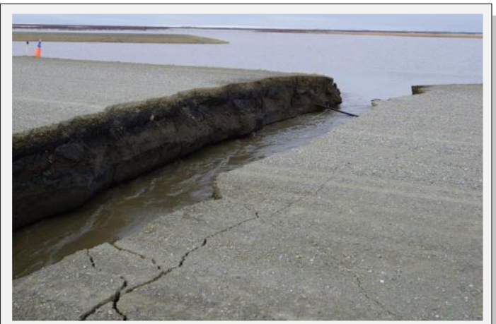
A 50-foot wide section of the Emmonak Airport taxiway was washed out and electrical and communication lines damaged by Yukon River spring flooding.
