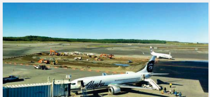
Construction projects were in full swing last summer at ANC - including reconstruction of Taxiway E2 (above), Taxiway M, Taxiway L, and Runway 7L.
