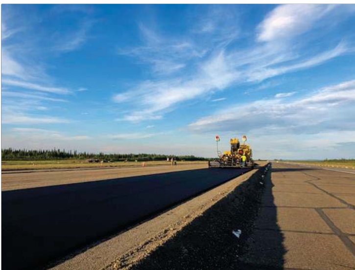
Galena Airport's runway is paved under some beautiful summer weather. Photo thanks to Larissa Figley, DOT&PF Engineering Technician.
