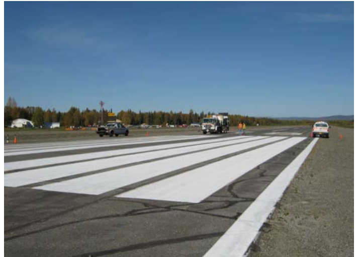
Runway maintenance at the airport includes crack sealing, paving, painting and lighting repair.
