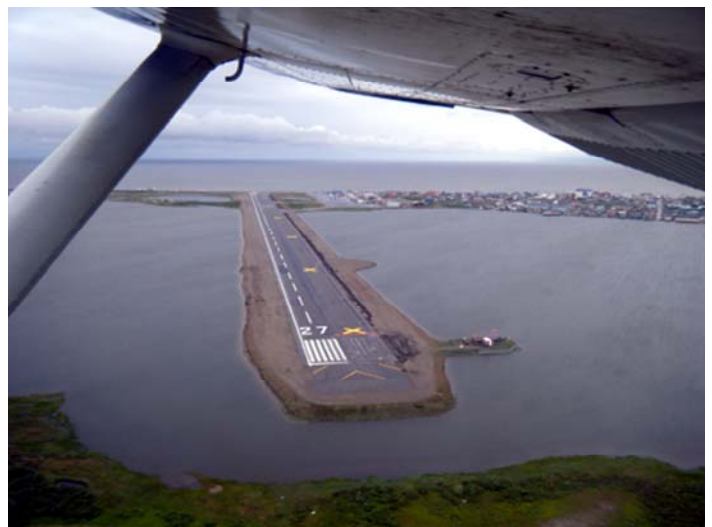
The Kotzebue Airport maintained operations with half of the runway closed for construction work.
