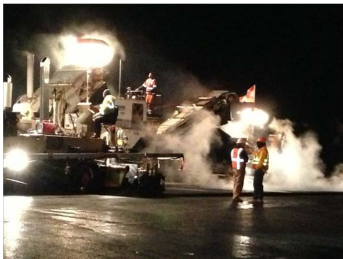
Night time paving operations at the Sitka Airport. (Photo courtesy—Maureen Hanson, DOT&PF)
