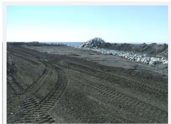
The new access road around the west end of the Kotzebue Airport main runway under construction
