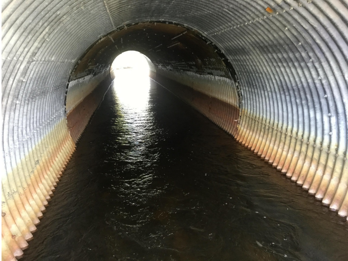
Figure 1: Caswell Creek joint separation, looking downstream
