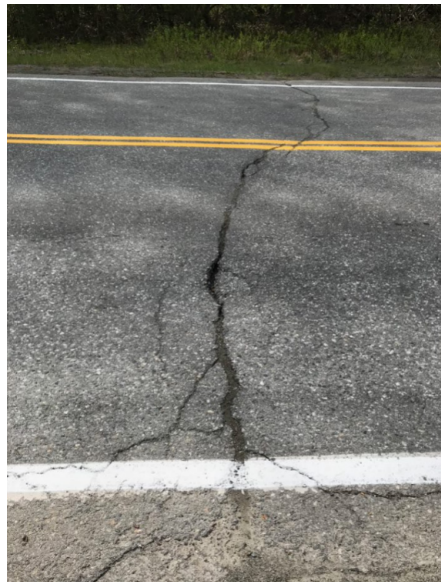
Figure 1: Transverse cracking along Clark-Wolverine Road
