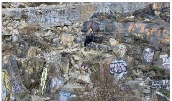
The Exterior of the Summit Tunnel. Without any federal, state, city or county markings to denote and protect its historic significance, the site has been vandalized with graffiti. Forgotten are the 20,000 Chinese immigrant workers who sacrificed for this infrastructure, linking the United States from east to west coast.
