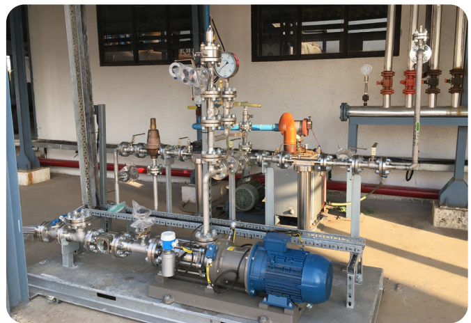
CEHB sealless magnetically coupled side channel pump installed in Koura's filling plant. Pump is equipped with level controller and a Detect sensor for vibration monitoring.
