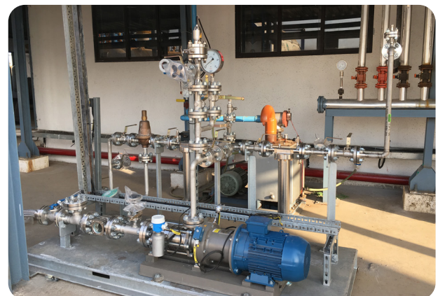
CEHB sealless magnetically coupled side channel pump installed in Koura's filling plant. Pump is equipped with level controller and a Detect sensor for vibration monitoring.
