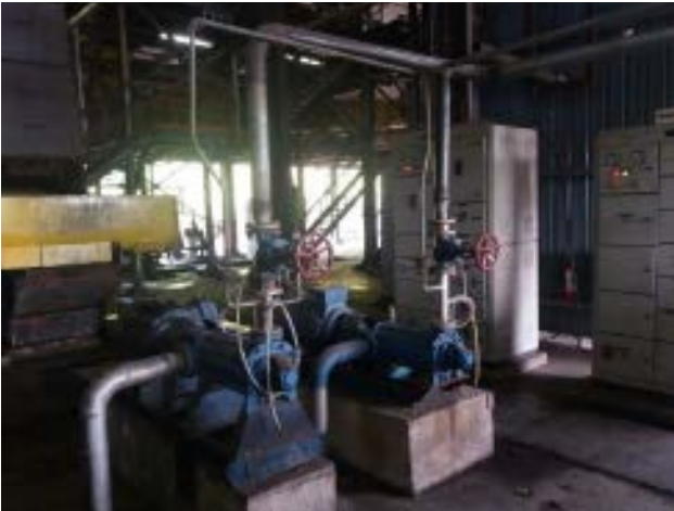
Boiler feed pump (SIHI model HEGA multistage)
