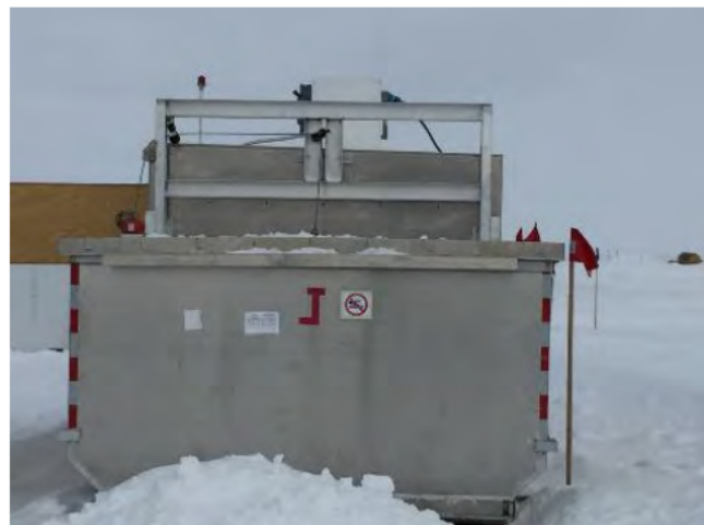
Existing Snowmelter Used to Make Potable Water
