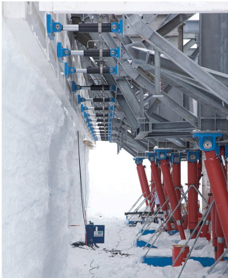
Figure 11. Numerous hydraulic jacks (blue and black color at upper left of photo) allow the apron to engage the snow alongside, thereby distributing horizontal wind loads on the elevated building into that snow. Note the vertical bipods are visible at the lower right of this image (Gernandt et al. 2010).
