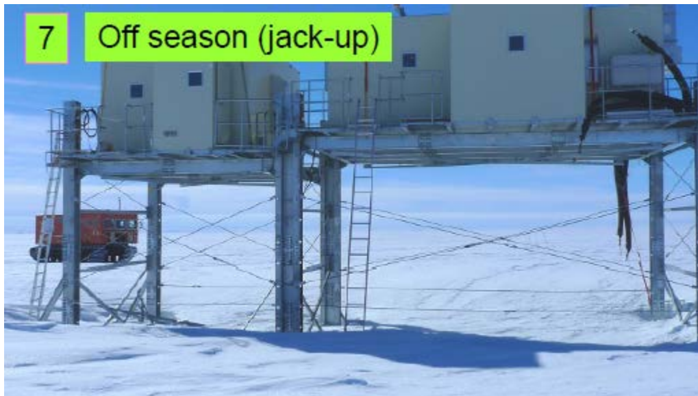
Figure 21. Jackable shelter near Syowa Station, Antarctica (courtesy of K. Ishizawa, Japan NIPR).
