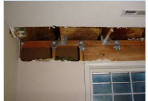
Adding hurricane straps from inside a house requires the removal of wall and ceiling finishes. Stronger connections also are needed at the base of the wall.
