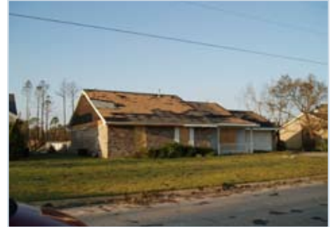
The loss of roof cover and underlayment can lead to significant water intrusion.
