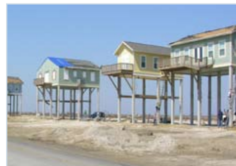
Figures 29 and 30 Ground level views, looking west, of the Fortified houses before and after Hurricane Ike. It is clear that all storage areas and decks were totally destroyed by the storm surge.
