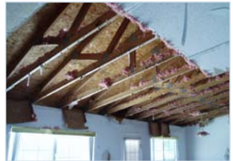
Collapsed ceiling due to water intrusion from roof cover damage.
