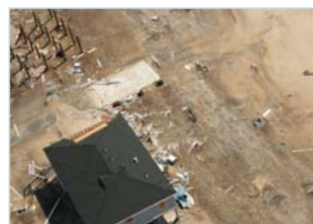
Figure 28 Gable end failures, and particularly of roof sheathing loss at gable ends, were a frequent source of damage. In several cases, it was clear that outriggers supporting sheathing had been notched, and in some instances, underlying rafters or trusses also probably were notched.
