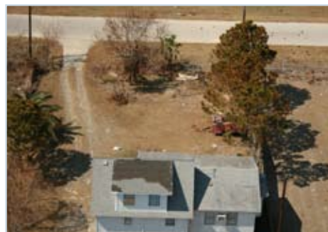
Figure 24 In many cases of roof damage, underlayment survived during hurricane conditions where shingles did not.
