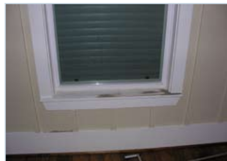
Figure 38 Water got inside this window, despite the presence of a hurricane shutter and the use of impact-resistant glass.
