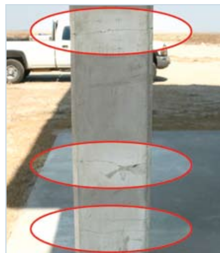
Figure 32 These horizontal cracks are indicative of the columns experiencing large tension forces from uplift on the decks when they were impacted by the storm surge with waves. If the cracking had been due to lateral loads, it would have produced diagonal cracks across the cross-section.
