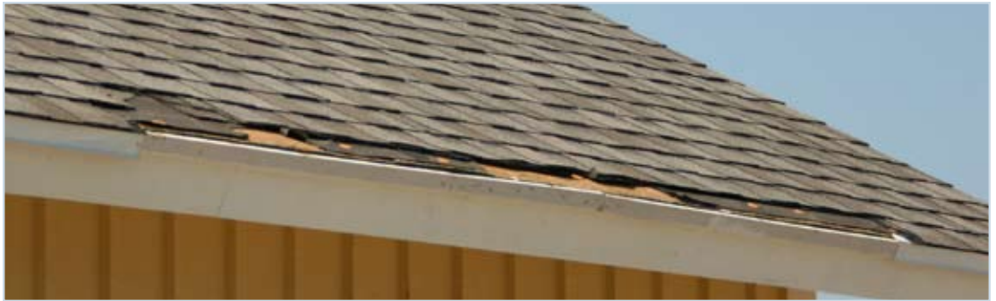
Figure 35 Drip edges may be vulnerable to corrosion and may play a role in eave shingle failures when they are not attached with enough fasteners. In this photo, the drip edge is deflected upward and may have contributed to the lifting of shingle tabs immediately adjacent to the eave.
