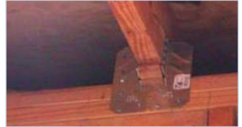
Add hurricane straps to tie the roof structure to the walls from the soffit area.
