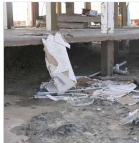
Figure 18 The concrete slab at ground level on the “Last House Standing” was significantly undermined by the effects of Hurricane Ike.
