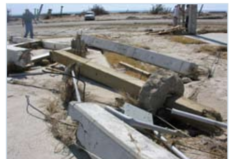
Figure 21 One of the porch columns from a traditionally built house across the street from the Fortified homes on Bolivar Peninsula. Some of the posts that broke away from the houses damaged by storm surge became sizeable battering rams, capable of damaging surrounding properties.
