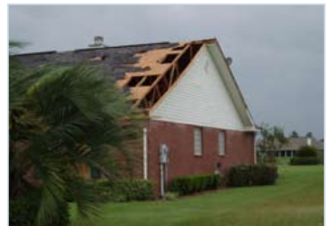
Loss of roof sheathing allows water and wind inside.
