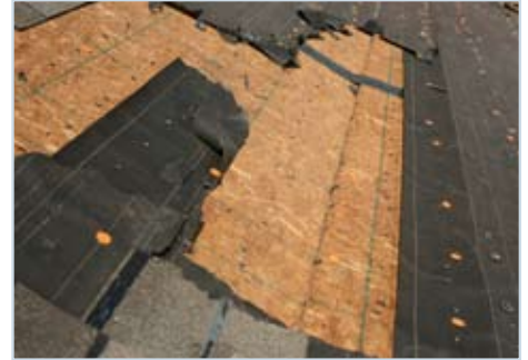
Figure 25 Flashing should have been installed at the joint where OSB sheathing panels overlapped on the primary slope of this traditionally built home, beginning at the ridge. This picture clearly shows that water collected and ran down through the gap between the sheathing.
