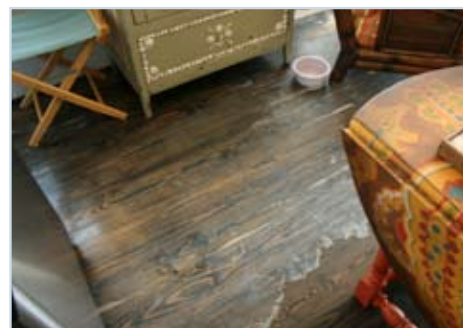
Figure 39 The silt line on the floor on this home is evidence of just how much water got inside. The use of water-resistant materials, such as wood flooring, prevented widespread water damage.
