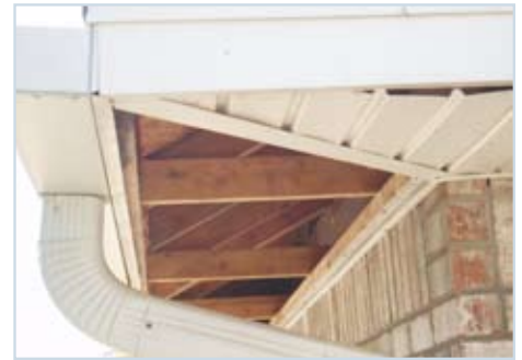
Loss of soffit materials allows wind and water to be blown into an attic.
