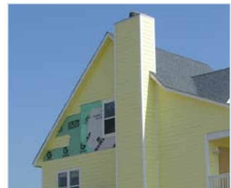
Figure 17 The “Last House Standing” was missing exterior wall cement board panels on both the seaward and inland sides of the home.
