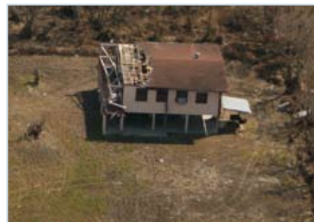
Figure 27 Losses of roof sheathing at gable ends were frequently observed toward the western end of the Bolivar Peninsula, where the 3-second gust wind speeds were likely less than 110 mph.
