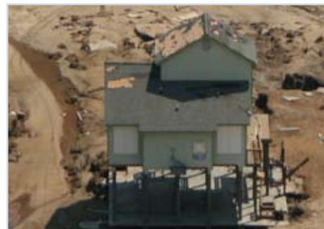
Figure 26 The 15-pound felt underlayment in this home did not survive hurricane conditions after the shingles were lost. This problem was addressed in the Fortified homes through the use of tape over the seams to provide backup water protection.
