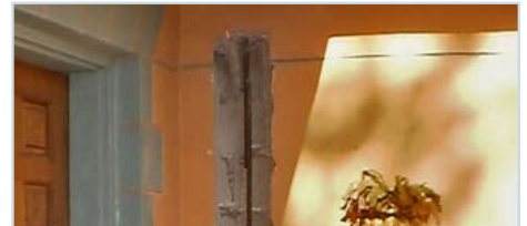
Adding steel can strengthen and reinforce a masonry wall and provide a continuous load path.
