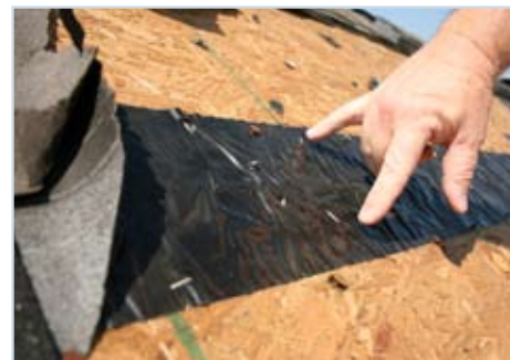
Figure 33 Here staples were used in an apparent attempt to keep the secondary water barrier tape in place, likely due to the fact that the tape was not sticking well when it was first applied.
