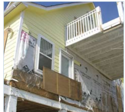
Figure 16 The wall of the first habitable floor on the seaward side of the “Last House Standing” had begun to fail when IBHS inspectors visited the site.
