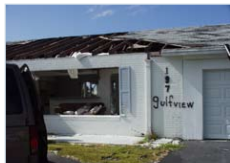
The large porch on this house was blown away and left a large hole in the main roof.
