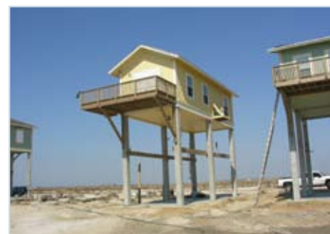
Figure 31 While all of the decks did break away, it is clear that deck connections were not what typically would be considered a breakaway connection in the Coastal Construction Guidance from FEMA and the NFIP.
