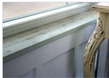
Figure 37 Even during a Category 2 hurricane, where rainfall rates never exceeded a rate of about 1 inch per hour, wind-driven rain leaked into the house through windows and doors.
