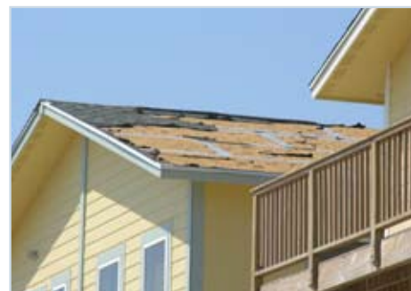
Figure 34 Workers opted to use a different type of secondary water barrier tape than was used on one of the last Fortified houses in the row on Bolivar Peninsula.
