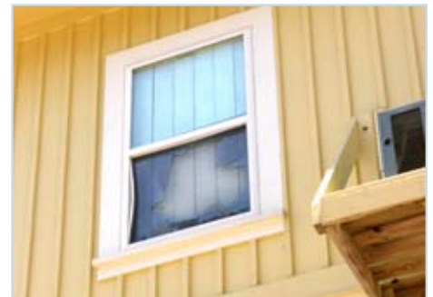
Figure 36 Only one outer pane was broken and no inner panes were damaged on the impact-resistant windows used in the 10 Fortified houses that survived Hurricane Ike.
