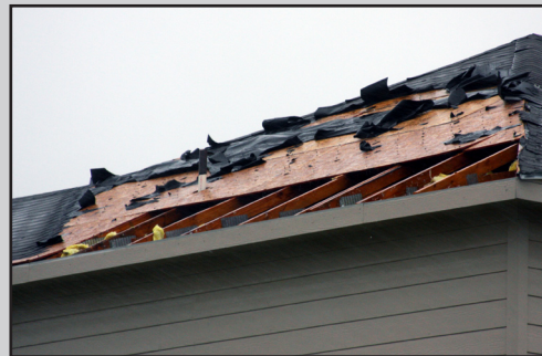
HEAVY DAMAGE AS A RESULT OF SHINGLE AND SHEATHING LOSS
