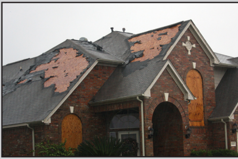
WIDESPREAD DAMAGE TO ROOF SHINGLES
