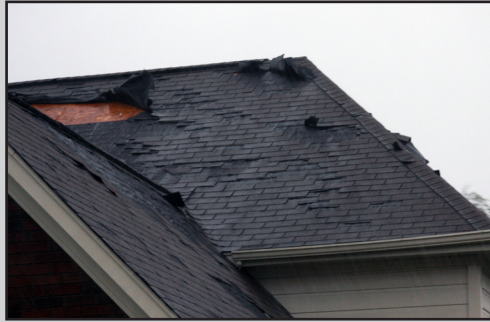
A LARGE NUMBER OF SHINGLES BLOWN OFF
