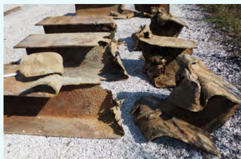
Failed pile sections
