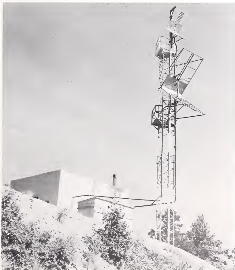
Closeup view of antenna tower at "base site," Cheyenne Mountain, showing details of the 92-MHz and 210.4-MHz (later modified to 236 MHz) transmitting antennas. The structure housing the transmitters is at the left.
