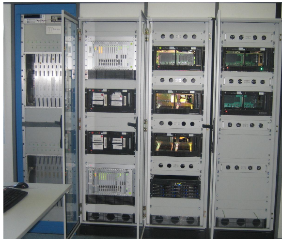
Figure 1. Left-most rack contains the two correlator crates. Rack second from left contains two station units with two rack-mounted Mark 5A playback units. Rack second from right contains from top to bottom three Mark 5B units and the eVLBI-dedicated linux computer. Right-most rack contains two Mark 5B units.
