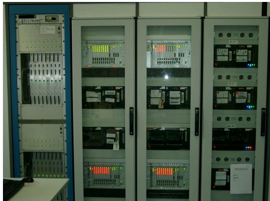
Figure 1. The left-most rack contains the two correlator crates. The racks second and third from left contain two station units with two rack-mounted Mark 5A playback units. The right-most rack contains three Mark 5B units and a Mark 5A unit dedicated for e-VLBI.
