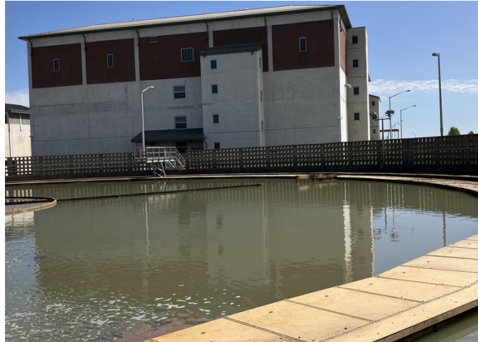
Image 03: Clarifier #4, missing section of skimmer arm.
