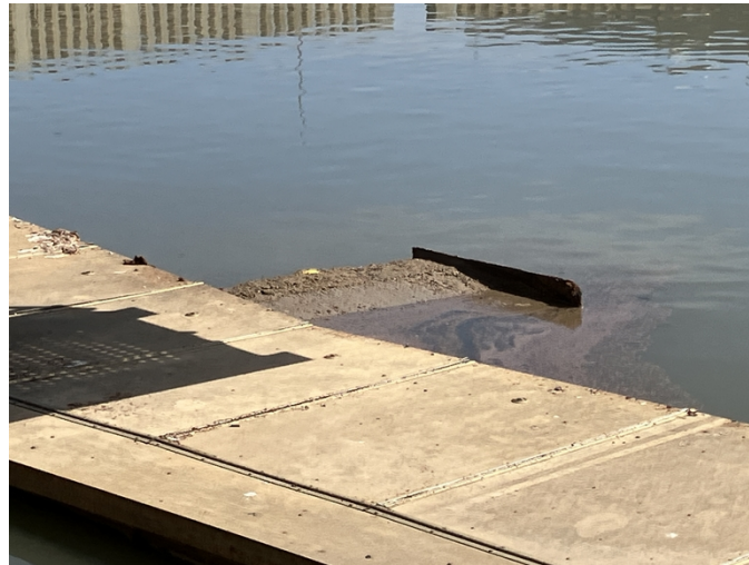
Image 04: Clarifier #4, clogged scum trough.
