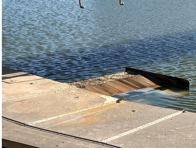
Image 5: Clarifier #2, Clogged scum trough.
