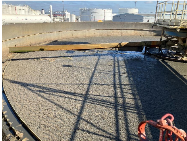
Image 2: GST #1, Broken & missing skimmer flaps.
