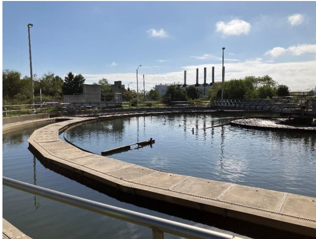
Image 6: Clarifier #5b, Bent skimmer arm.
