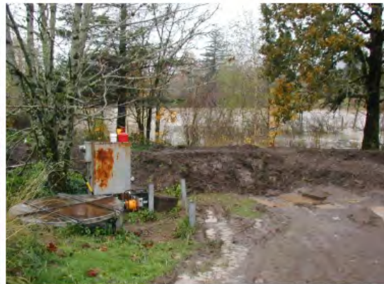
City Wastewater Pump Station Greenleaf Lake East Shore
