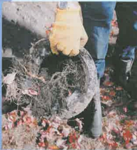
Tree roots are a common cause of clogged side-sewer lines. Roots can easily penetrate pipes made of porous concrete such as this one, which is more than 25 years old. Modern side-sewer lines are made of heavy duty, water-tight plastic and therefore last much longer.
