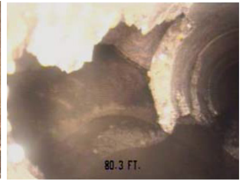
Large hole with void
