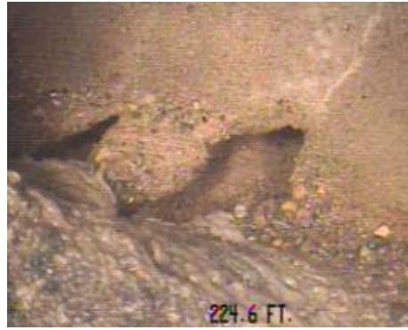
Medium hole with void
