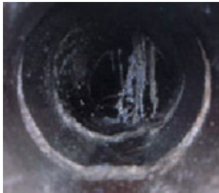
Clean groundwater pouring in through a defective joint.
