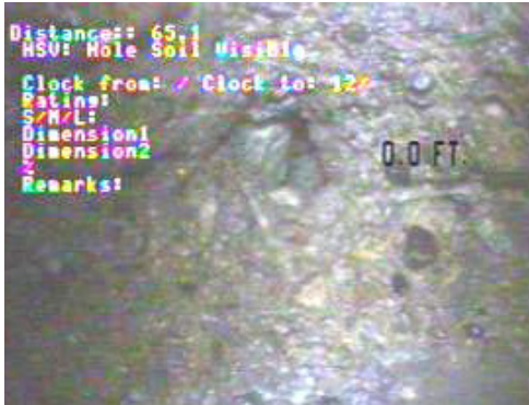
Small hole with aggregate showing
