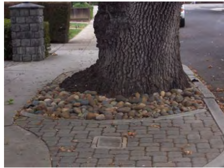
Roots offsetting curb and gutter; note: concrete edge band holding pavers
