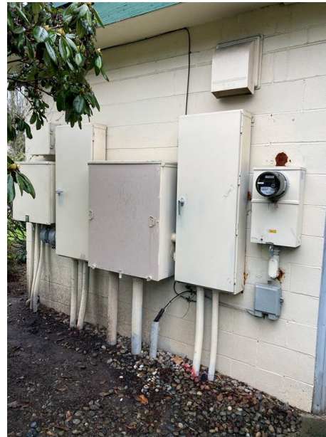
Protect and Maintain exterior electrical panels and CMU wall
