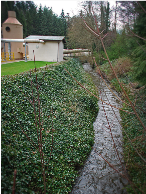
Figure 5.02 – Miller Creek, and the SWSSD-operated wastewater treatment plant.
