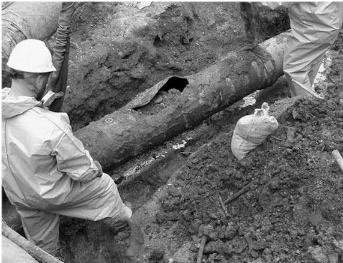
Figure 1: Ruptured 16" pipeline being removed from Whatcom Falls
