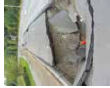
Deschutes Parkway failed along the entire corridor due to liquefaction during the 2001 earthquake.
