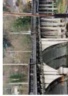
The Fourth Avenue Bridge in downtown Olympia was structurally damaged to vehicles immediately following the 2001 Nisqually Earthquake.
