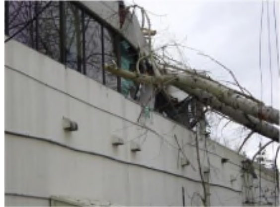
Figure 12. December 14th, 2006 Windstorm Kelsey Creek Shopping Center
