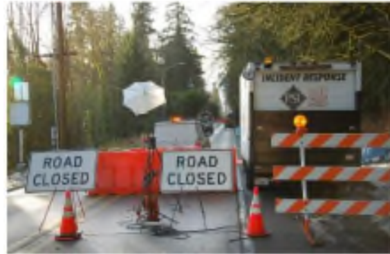
Figure 5. West Lake Sammamish Road Closed after Landslide in January 2012
