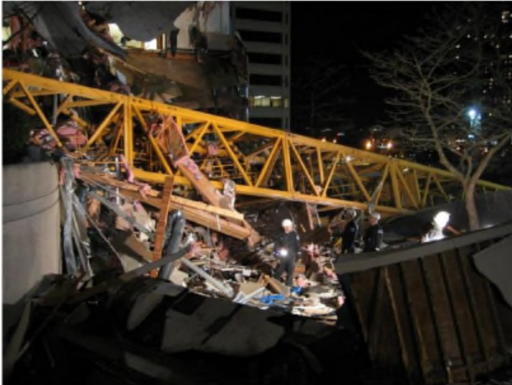
Figure 5. November 2006 Crane Debris
