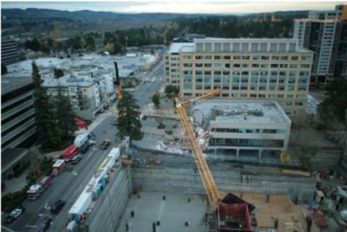
Figure 4. November 2006 Crane Failure
