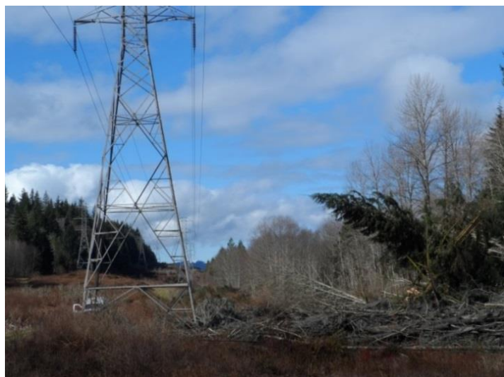
A steel tower of City Light's Skagit transmission line and debris deposited by the landslide near Oso, Wash. in March 2014. The debris caused minor damage to a tower.
