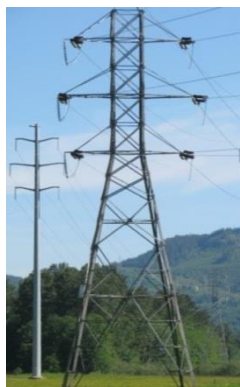
Transmission and Distribution
