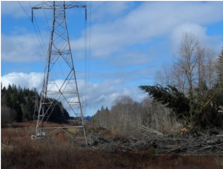
Photo: A steel tower of Seattle City Light's Skagit transmission line and debris deposited by the landslide near Oso, Washington in March 2014. The debris caused minor damage to a tower.
